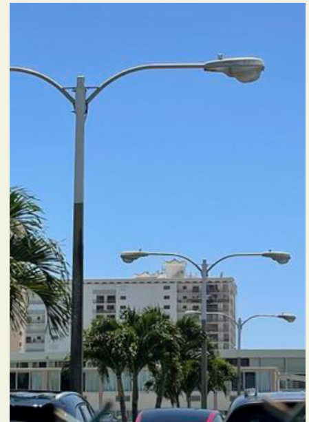
Larger scale streetlights typically found in auto-urban areas Source: Lighting Gallery
