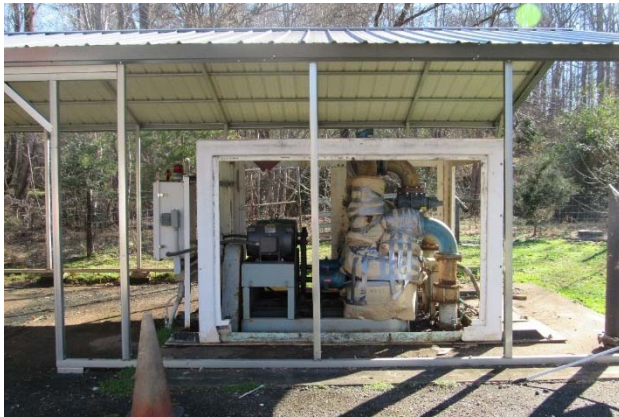
Figure 2.4 - Oxidation Ditch Aerators
