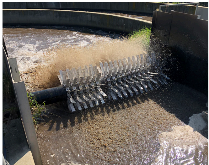
Wastewater Treatment Plant Oxidation Ditch
