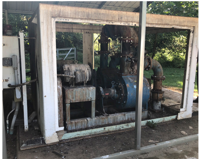
Wastewater Treatment Plant Influent Pump Station
