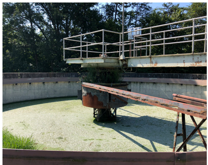
Wastewater Treatment Plant Clarifier
