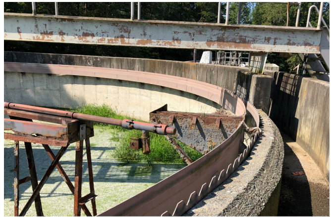
Wastewater Treatment Plant Clarifier
