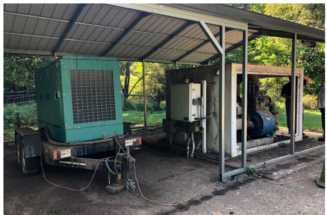
Wastewater Treatment Plant Influent Pump Station
