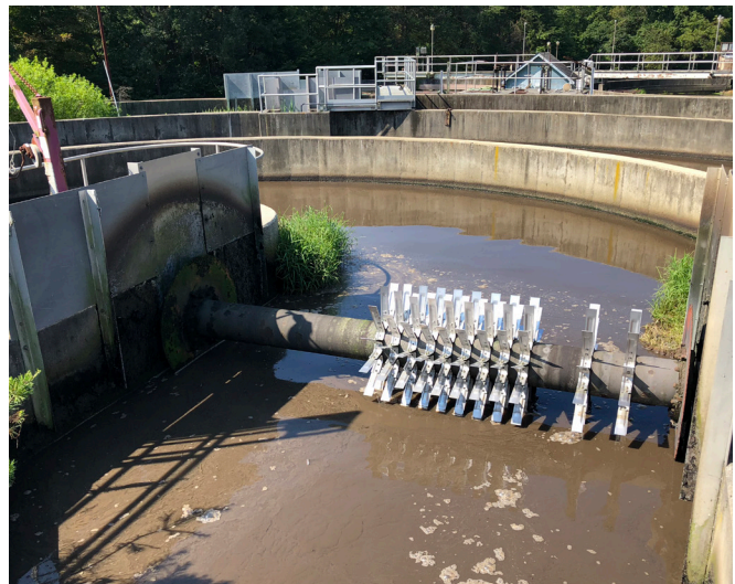
Wastewater Treatment Plant Oxidation Ditch
