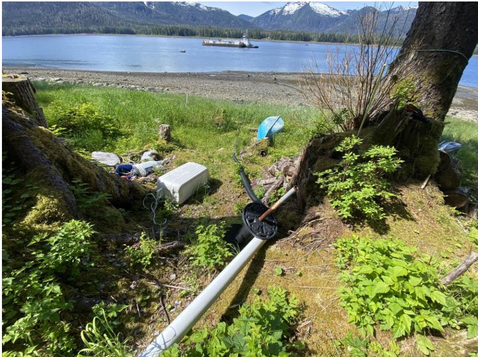
Pipe from septic tank going to beach.
