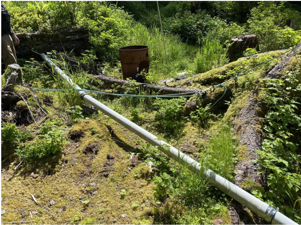
Pipe connected to septic tank.
