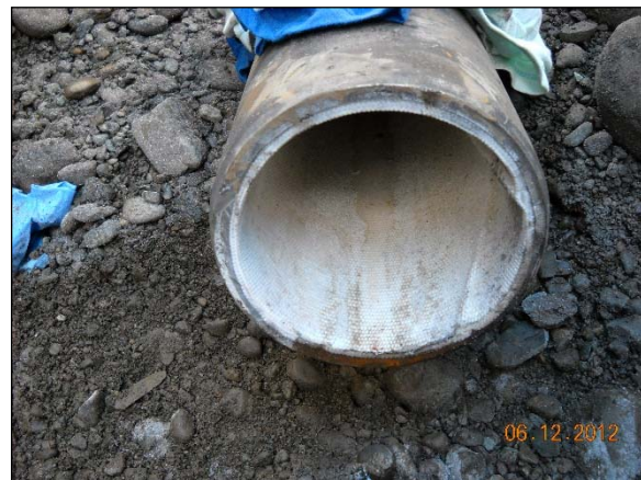
Figure 5: CIPP pressure liner in CI pipe
