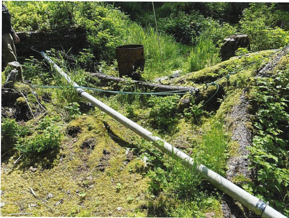
Pipe connected to septic tank.
