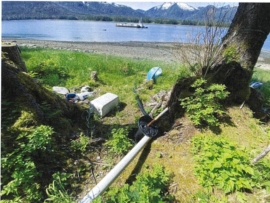
Pipe from septic tank going to beach.
