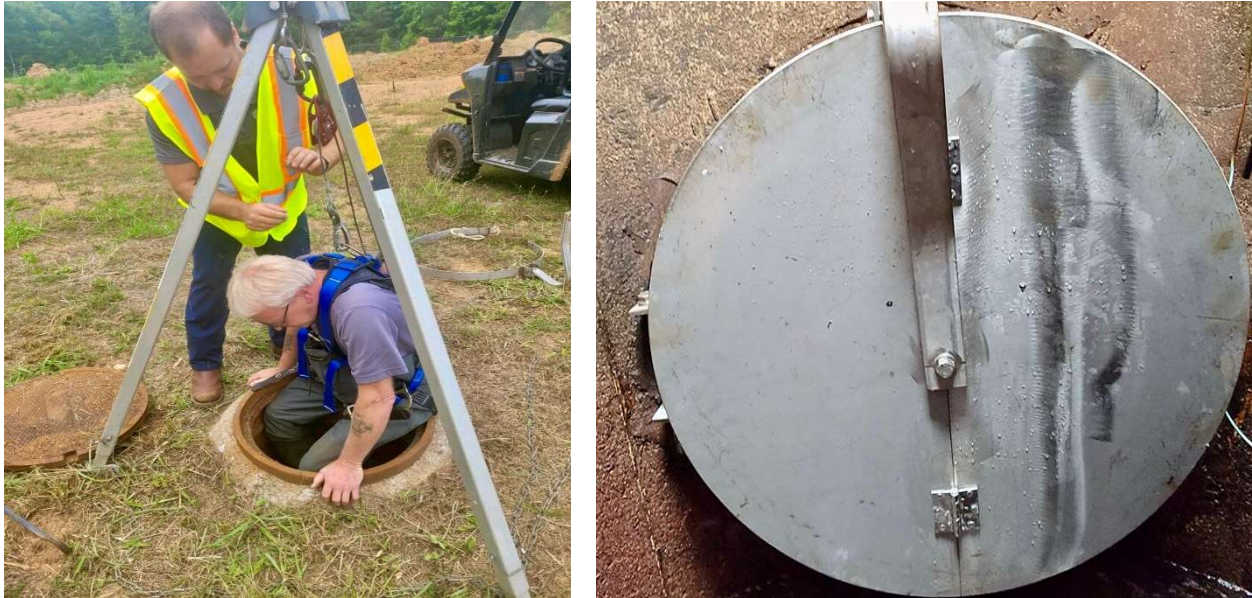
*Pictured above left: Will Spani conducts confined space entry. Right: 24" flapper valve installed.
