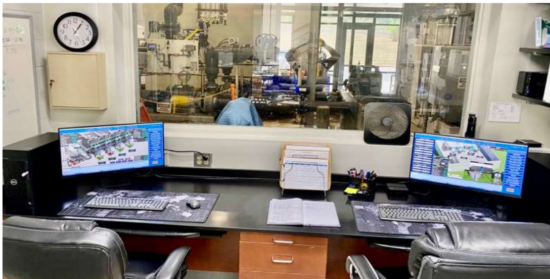
*Pictured above: New SCADA, well organized control room.
