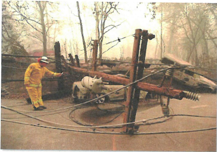
Pre-Fire Pole With PG&E Electrical Equipment
