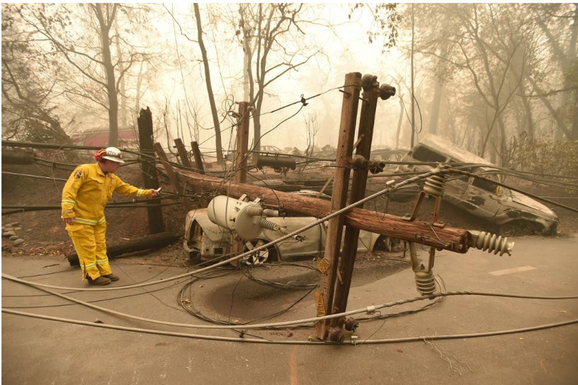
A burned utility pole crossing a Paradise evacuation route during the Camp Fire. Source: AP/Getty Images
