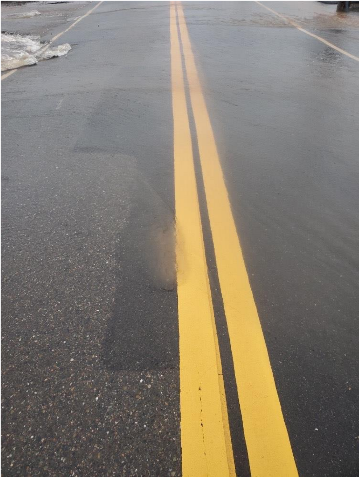
Figure 3 – Bille Road Flooding Over Roadway
