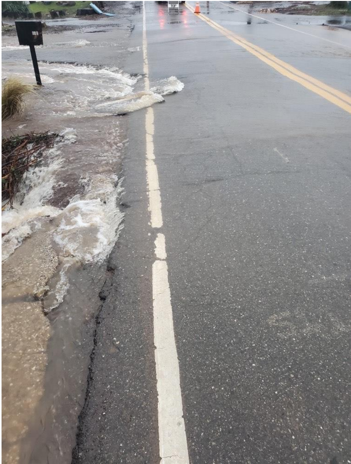
Figure 2 – Bille Road and Olympia Way Flooding
