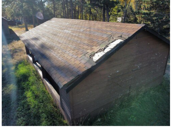
Replace damaged OSB.
