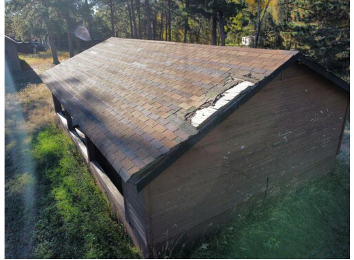
Replace damaged OSB.
