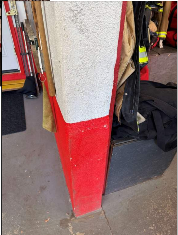
Photo 8: Demising wall between Bays #1 and #2. Likely 8" CMU that was the original exterior wall. Note concrete slab-on-grade floors.
