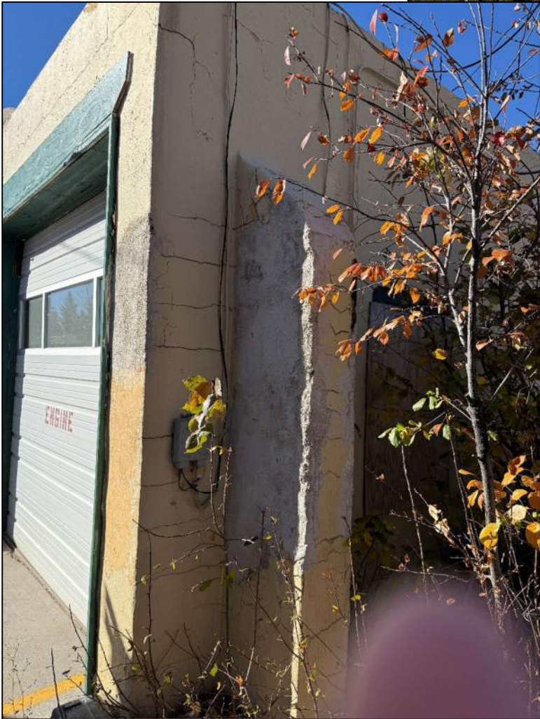
Photo 6: Northeast corner buttress. Lots of significant cracking in the plaster and patching that has occurred.
