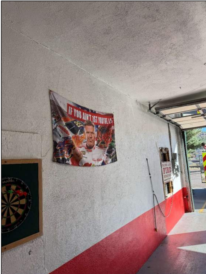
Photo 9: Interior north wall looking northeast. Note some minor cracking in the plaster mostly near a window infill.
