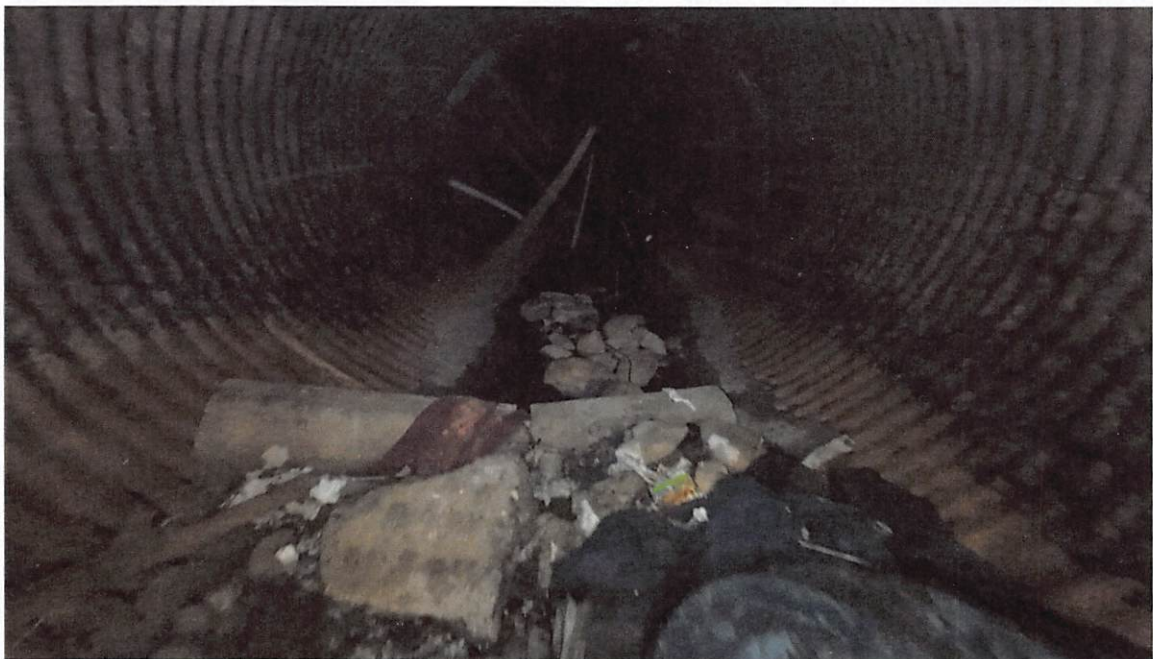
Trash pile and concrete in 72" Culvert
