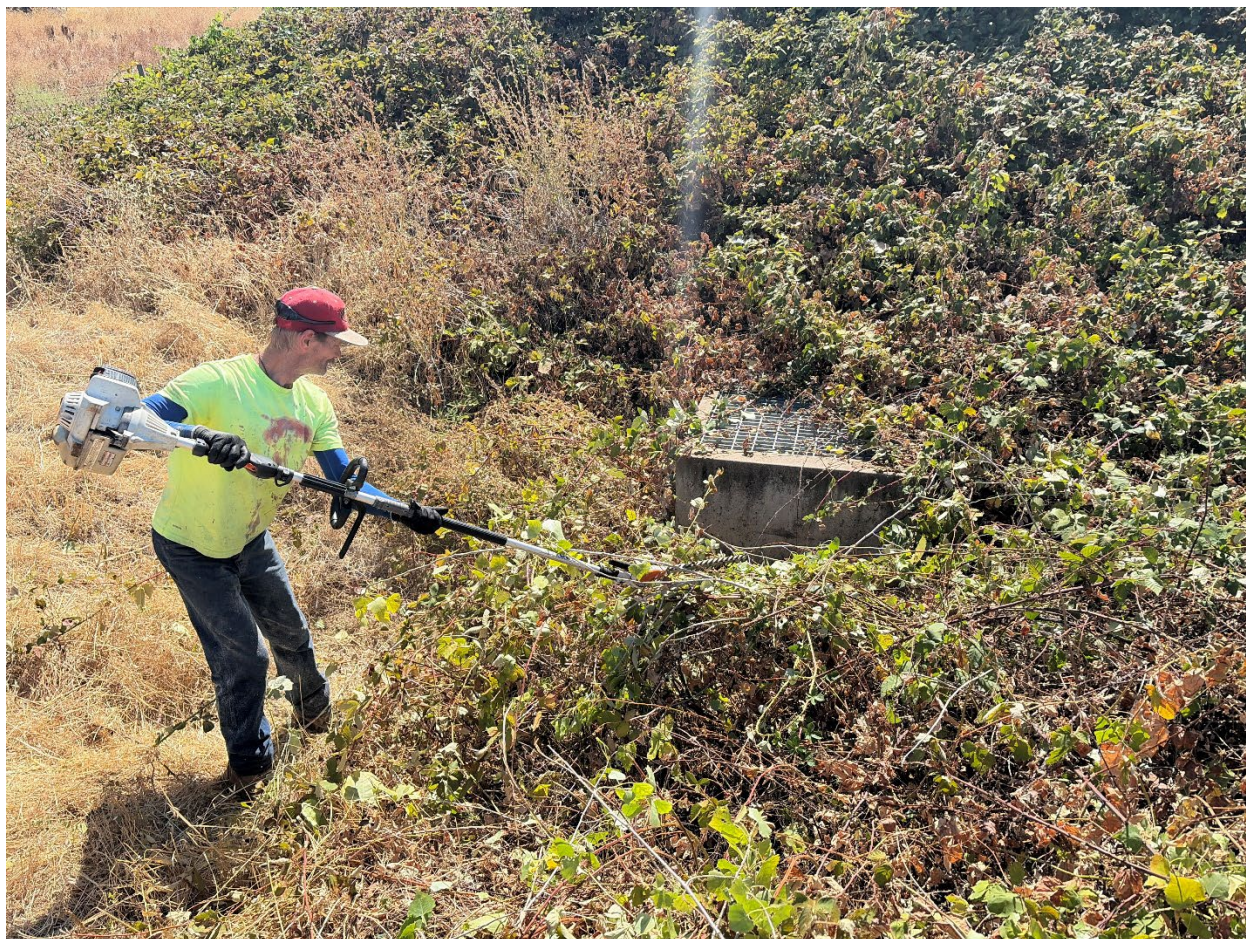
ABATEMENT OF VEGITATION CITY OWNED PROPERTY NEAR CAL WATER HEADQUARTERS
