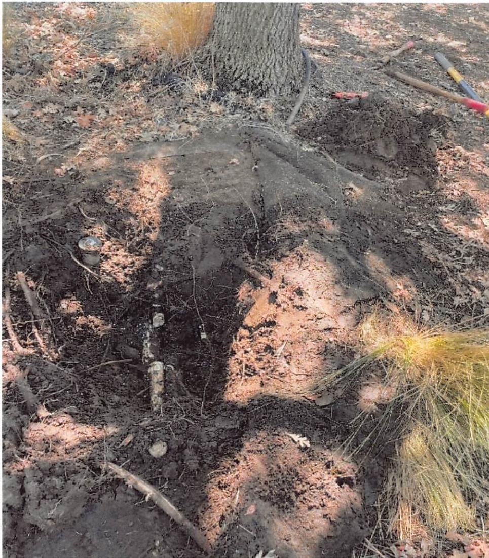
Broken sprinkler line caused by tree roots
