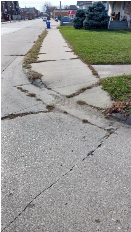
Non-compliant pedestrian curb ramp
