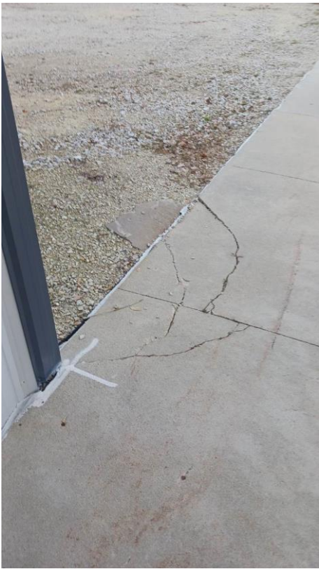
Severely broken PCC
