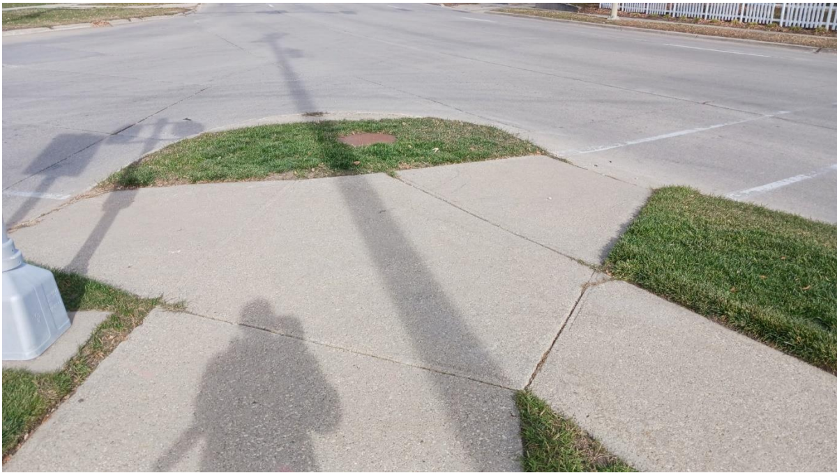
Non-compliant pedestrian curb ramp
