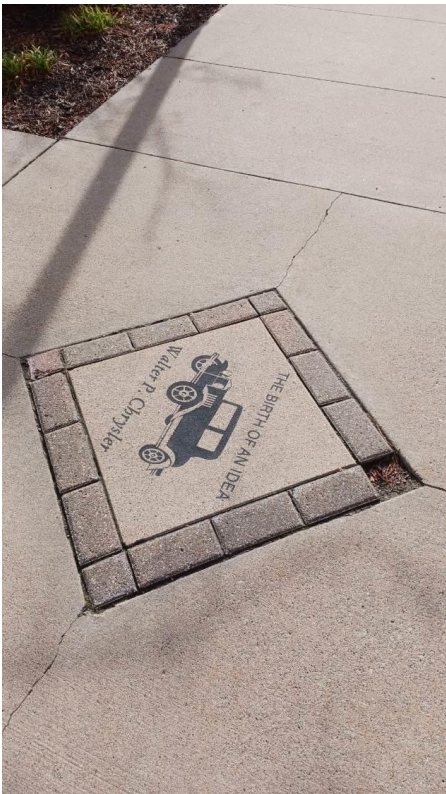
Missing paver causing trip hazard
