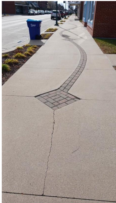
Settled pavers and diamond along with crack from end of diamond
