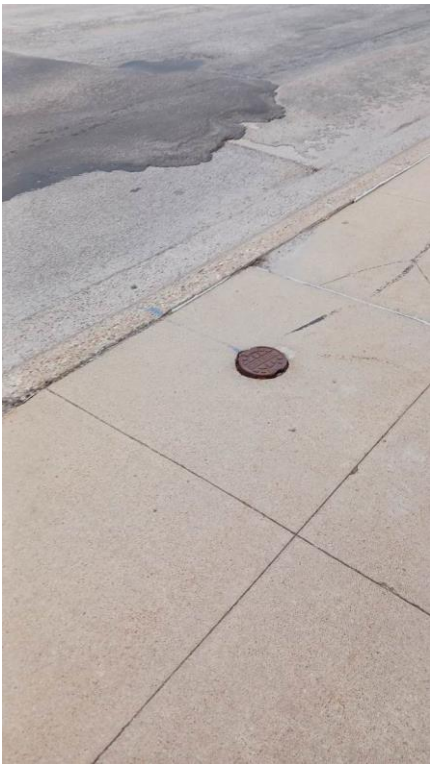
Protruding water valve
