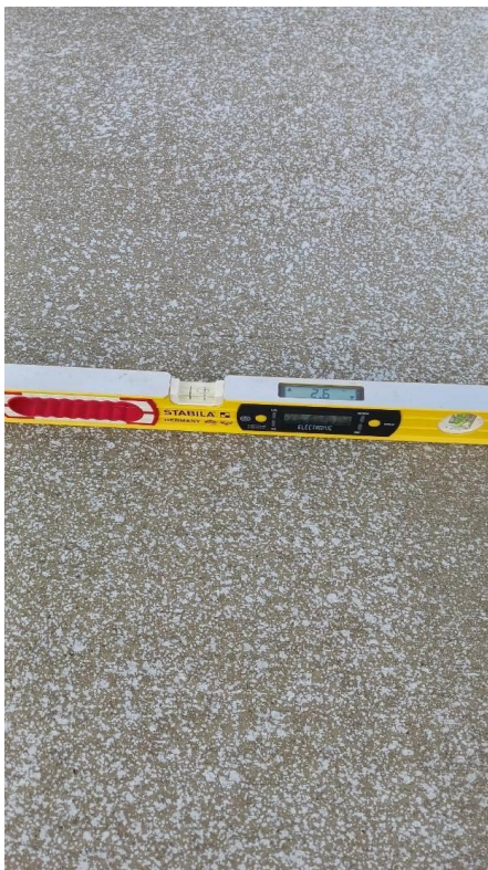
Cross slope greater than 2%
