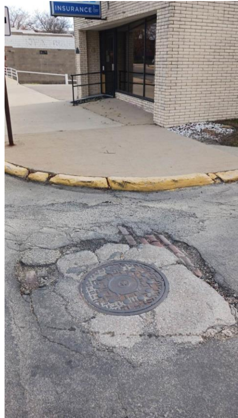
Non-compliant curb ramp
