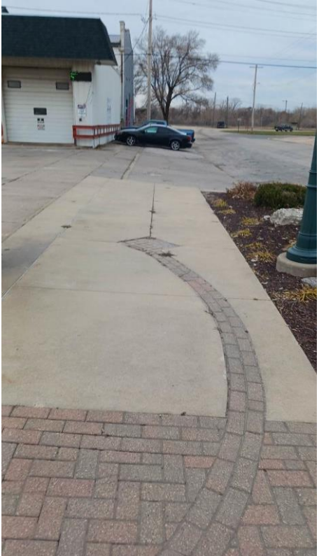
Cross slope greater than 0.25"
