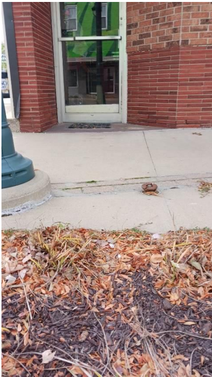
Protruding curb stop
