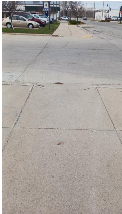
Non-compliant pedestrian ramp
