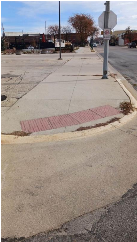
Curb height greater than 0.5"
