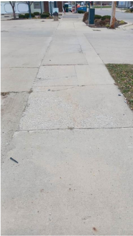
PCC displacement greater than 0.25"
