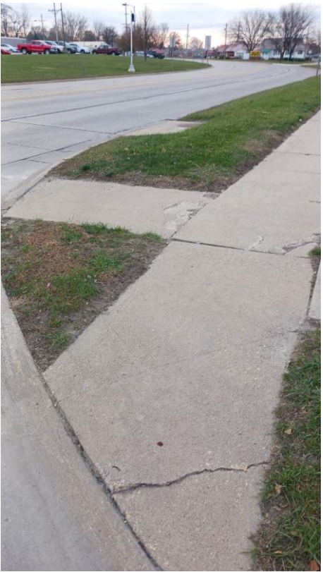
Non-compliant pedestrian ramp
