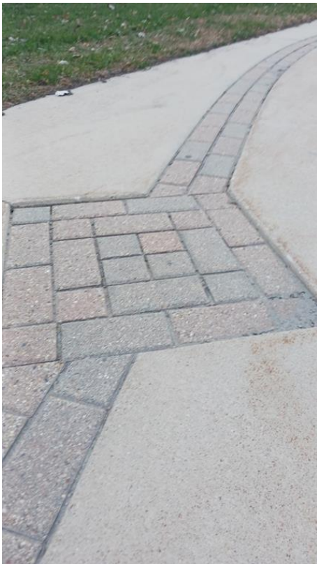
Paver settling, greater than 0.25"
