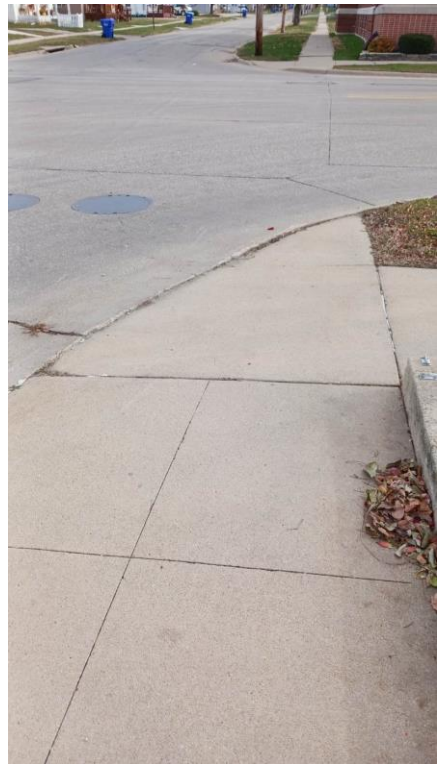
Non-complaint pedestrian curb ramp
