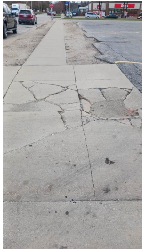
Severely broken PCC
