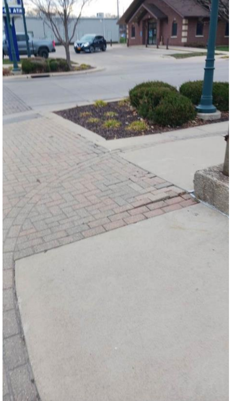
Heaving pavers with vertical displacement greater than 0.25"
