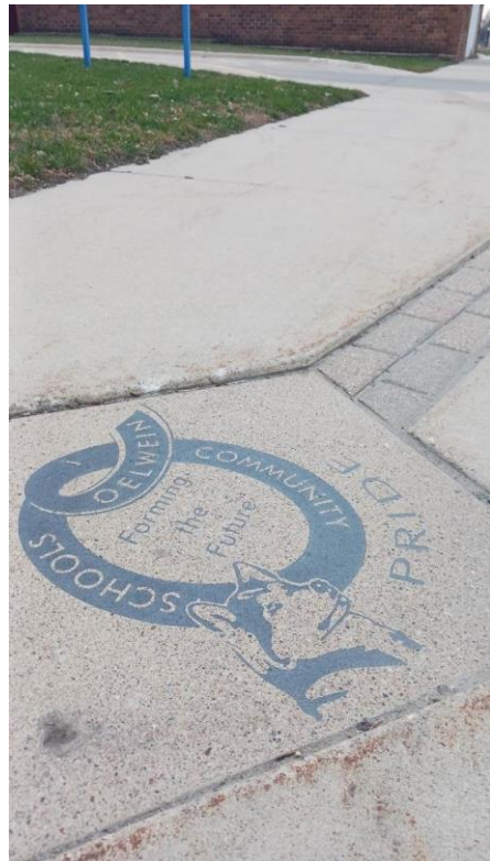
Paver and diamond settling, greater than 0.25"
