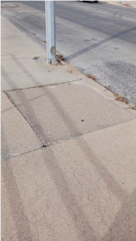
Settled PCC panel
