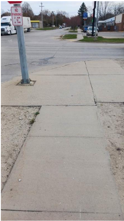
Non-compliant curb ramp
