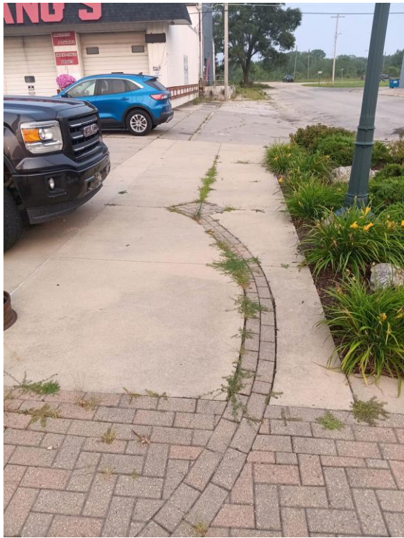
Vegetation in joints
