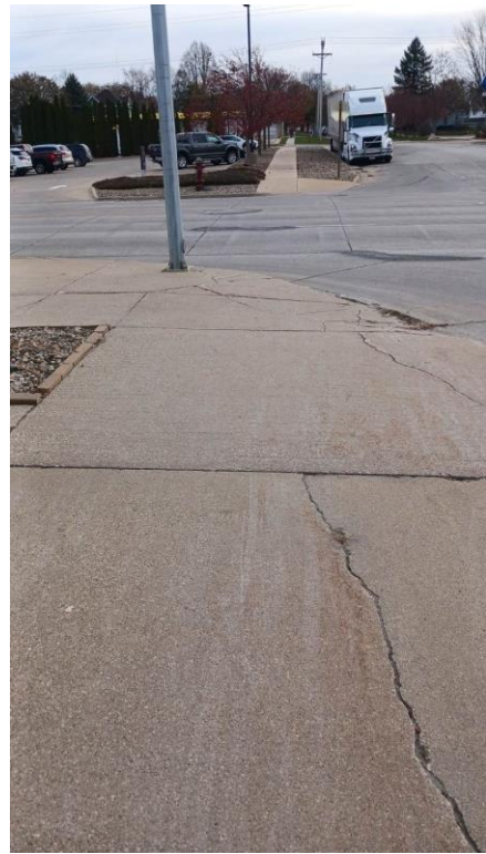
Non-compliant curb ramp
