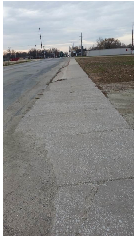
Cross slope greater than 2%
