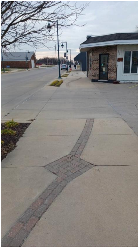
Paver settling greater than 0.25"
