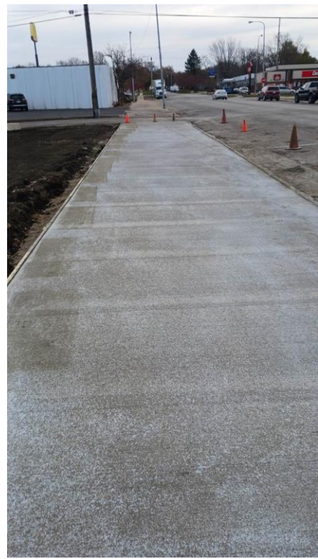
New sidewalk with greater than 2% cross slope
