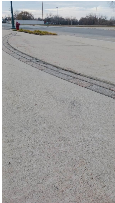
Pavement settling along paver band
