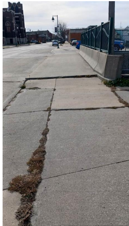
Vertical PCC displacement greater than 0.25" and cross slope greater than 2%
