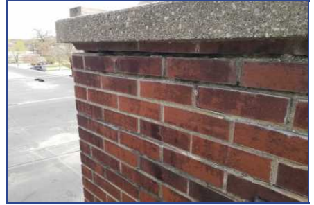
Section B - Deficiency #1 Chimney is falling apart causing leakage
