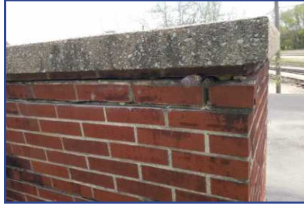
Section B - Deficiency #1 Chimney is falling apart causing leakage
