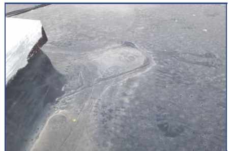
Section B - Deficiency #3 Membrane flashing voids, splits or open side flaps
