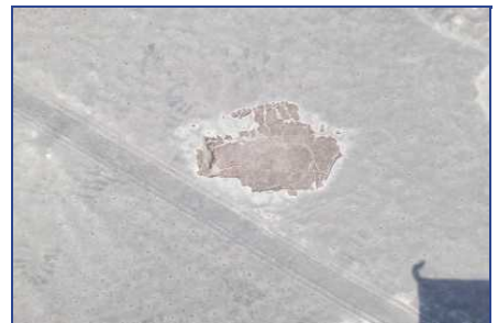
Section A - Deficiency #5 Failing caulking
