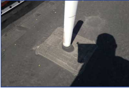
Section A - Deficiency #1 Pipe is flashed with a shingle roof seal
