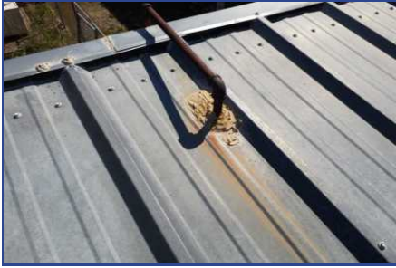
Section C - Deficiency #1 1" pipe coming through the roof is not flashed
