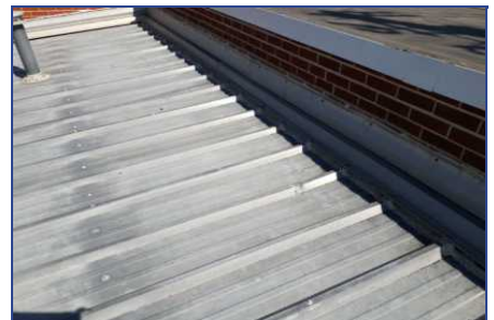
Section C - Deficiency #4 Foam gasket is deteriorated
