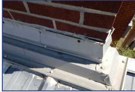
Section C - Deficiency #2 Metal flashing sealant deteriorated or missing
