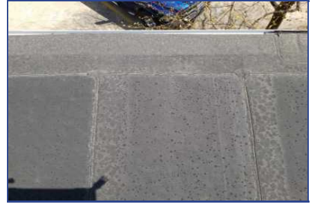
Section A - Deficiency #3 Open or Missing T-Joint patches
