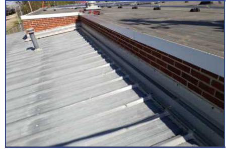
Section C - Deficiency #2 Metal flashing sealant deteriorated or missing
