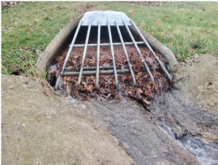
PLATT PARK INTAKE
