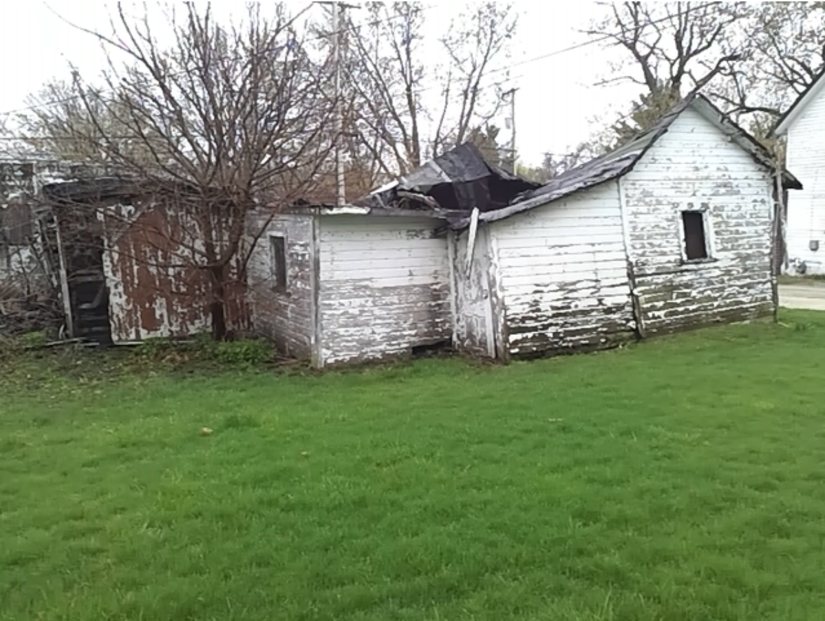
Photo: Collapsed Structure
