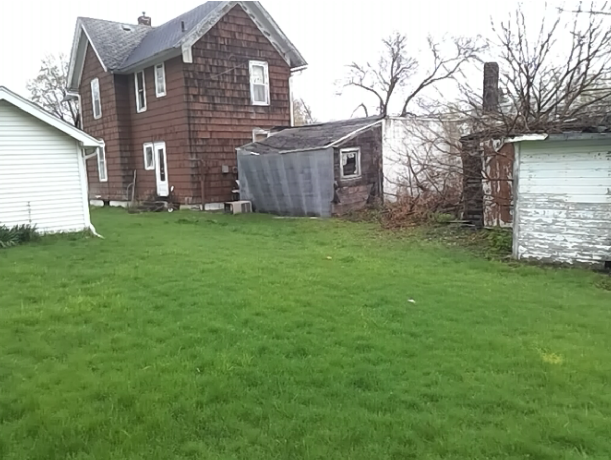
Photo: Collapsed structure
