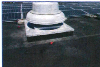
Section A - Deficiency #2 Void in patches
