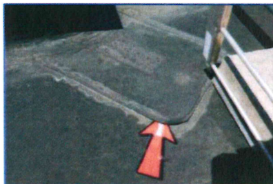
Section A - Deficiency #2 Void in patches
