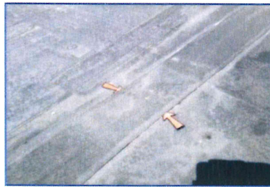
Section B - Deficiency #1 Voided patches over slices
