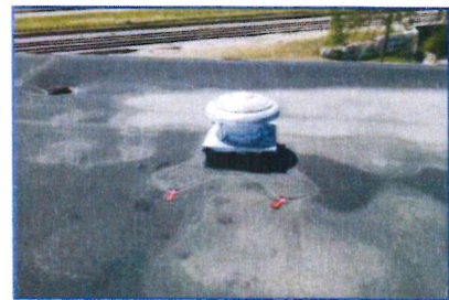
Section B - Deficiency #1 Voided patches over slices
