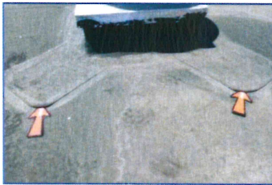
Section B - Deficiency #1 Voided patches over slices
