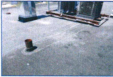
Section B - Deficiency #1 Voided patches over slices
