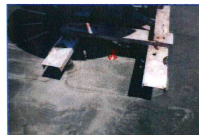
Section A - Deficiency #2 Void in patches
