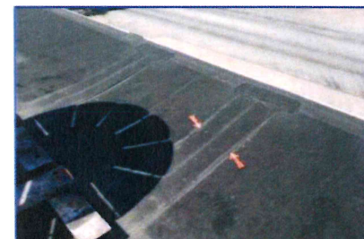
Section A - Deficiency #2 Void in patches
