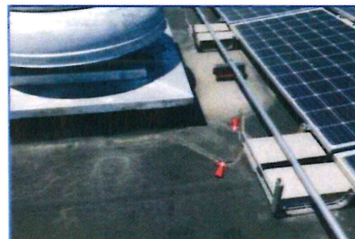
Section A - Deficiency #2 Void in patches
