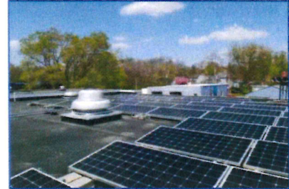
Section A - Deficiency #1 Missing slip sheets under each brick mount
