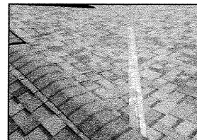
Section B - Deficiency #3 Deteriorated valley tin
