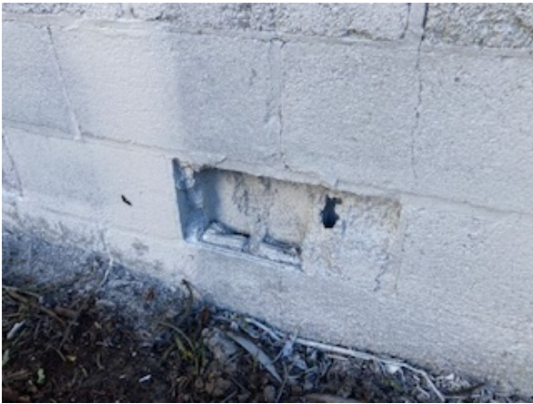
Foundation spalling near loading dock.
