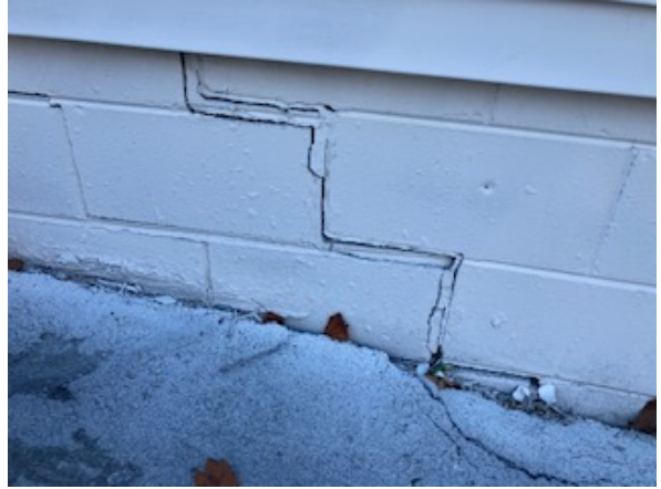
Example of minor settlement in front.
