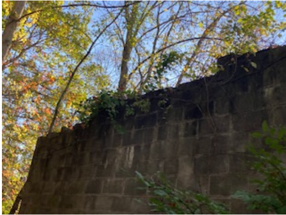
Spalling and missing blocks.
