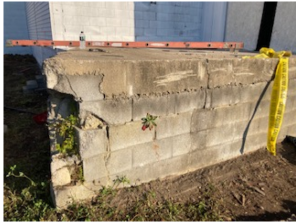
Loading dock cracks, spalling and settlement.
