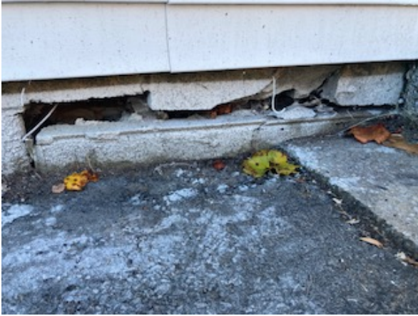
Damaged foundation in front.
