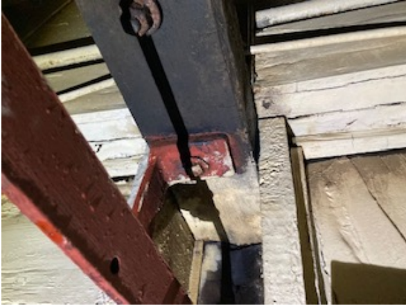
Rotted header above meat rack.
