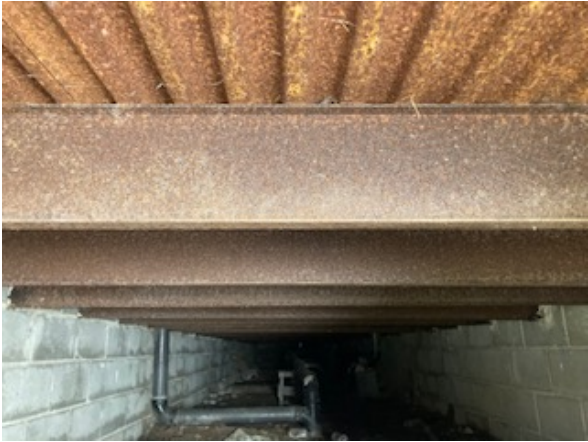
Rusted I Beams and decking.
