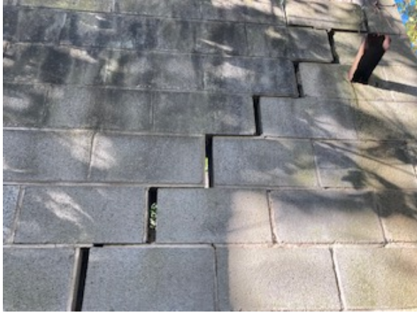
Train storage area wall with moderate settlement.
