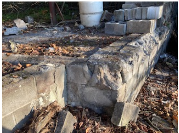
Retaining wall cracks, spalling and movement.
