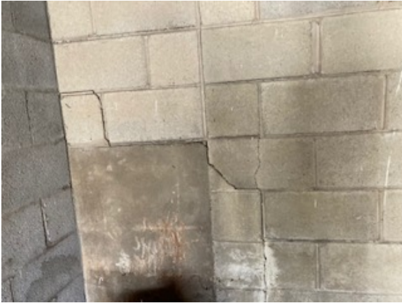
Example of minor settlement.
