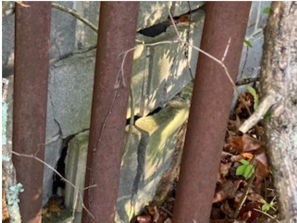
Foundation wall movement from tree roots.
