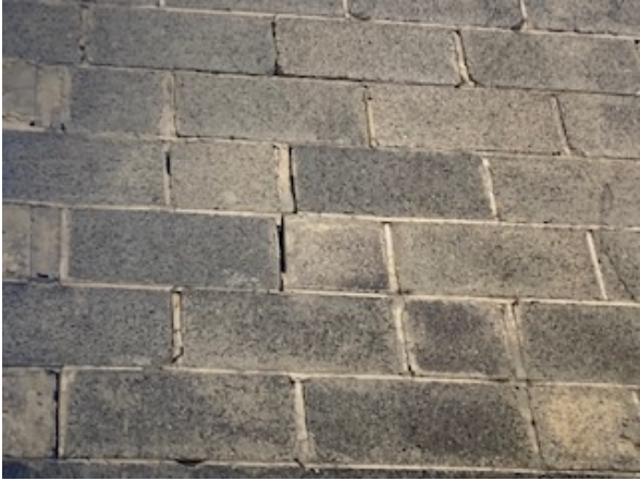
Missing grout in multiple areas of foundation walls.
