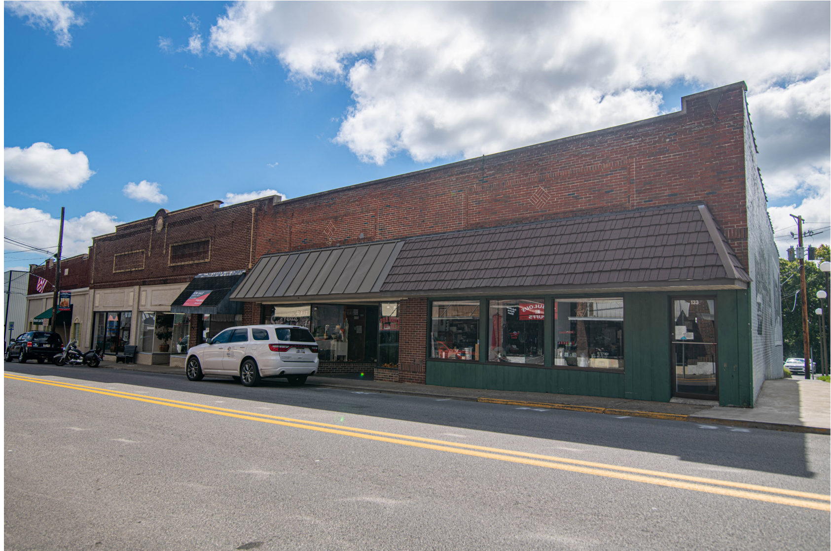
133 Main Street Canopies feel heavy and are mismatched. Facade brick at sidewalk level is covered with siding.
