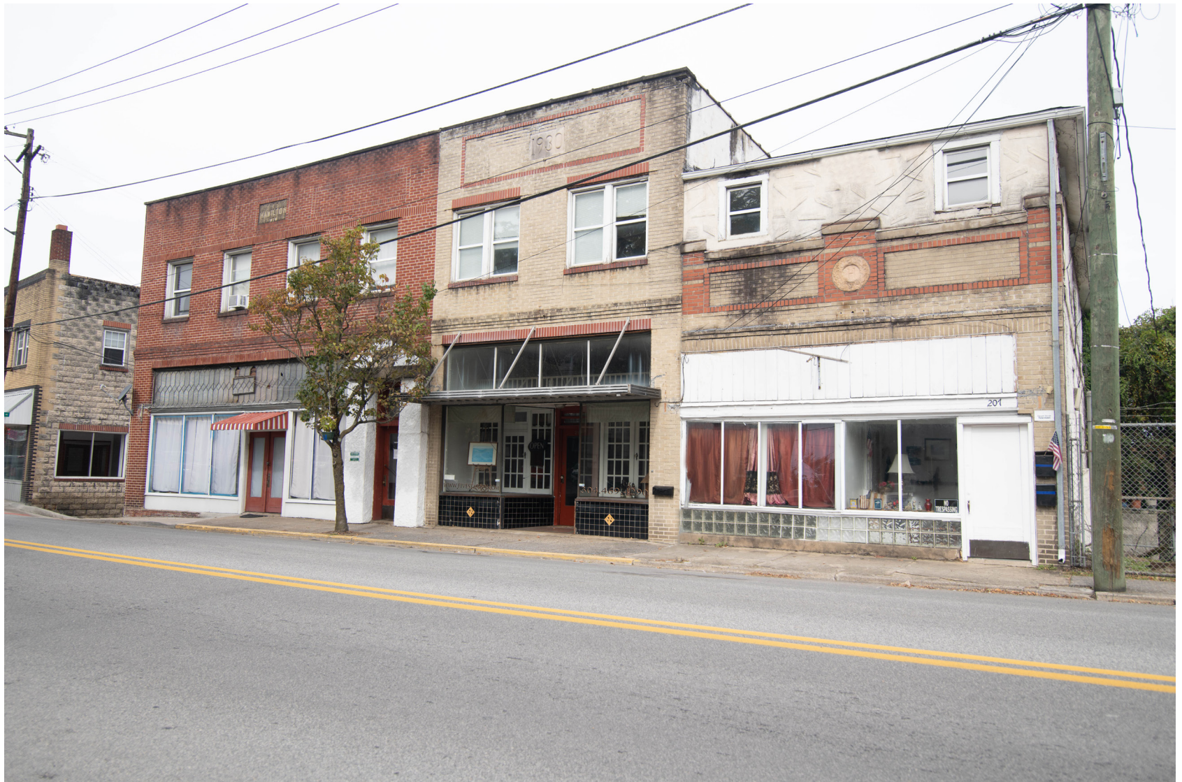
201 Main Street Addition to top of building is out of character. Brick is dirty. Lack of overall character.
