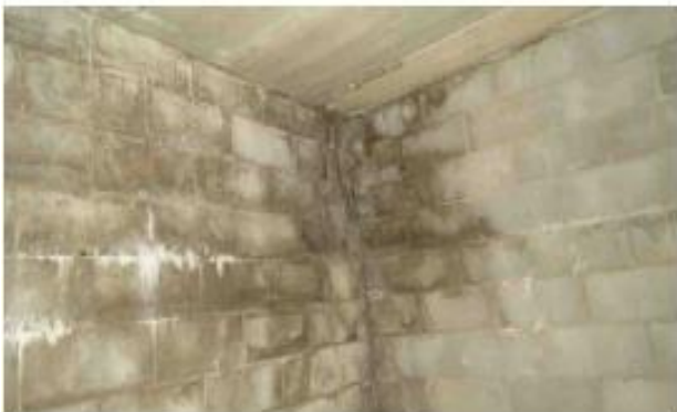
Previous Dampness in Basement
