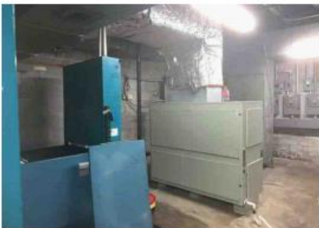
Electrical and Furnace Room
