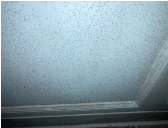
Probable mold on wall.
