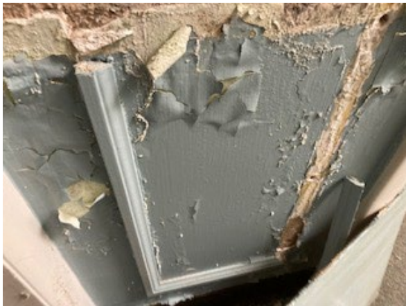
Evidence of prior bathroom leak.
