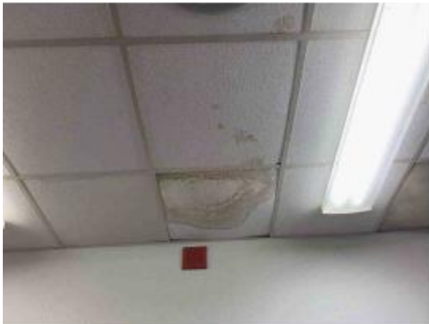
Damaged Ceiling Tiles
