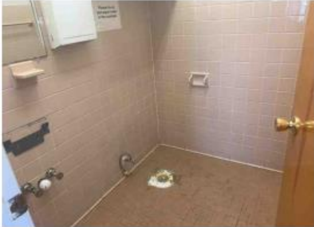
Non Working Restroom
