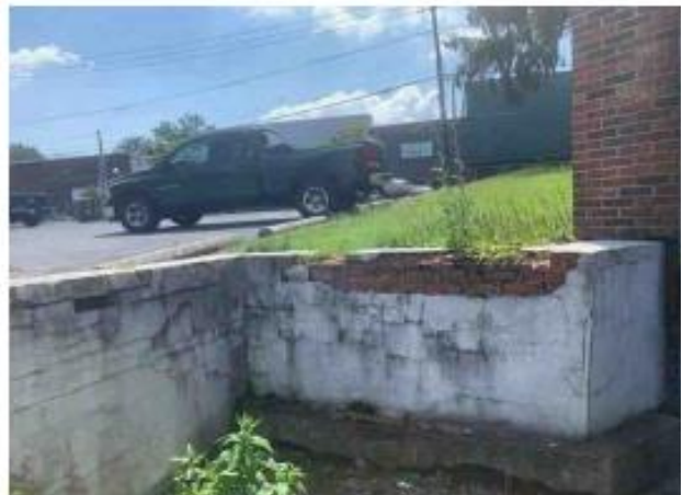
Retaining Wall Needs Repaired
