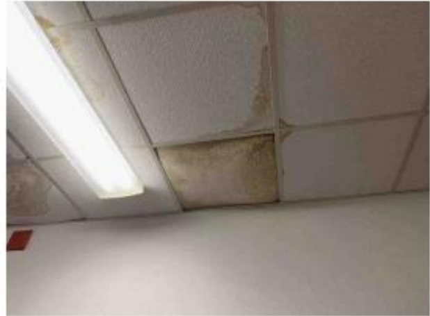
Damaged Ceiling Tiles
