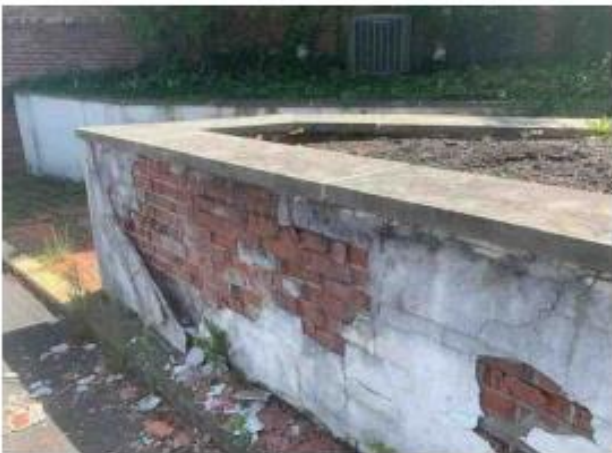
Damaged Retaining Wall
