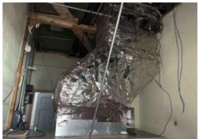
Duct Work from Furnace
