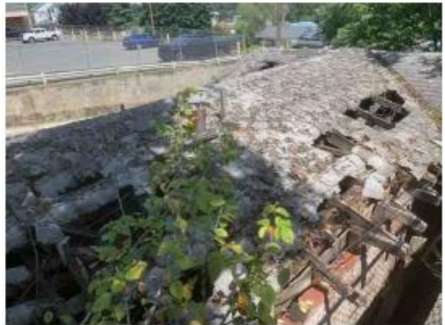
Deteriorated Roof on Garage Building
