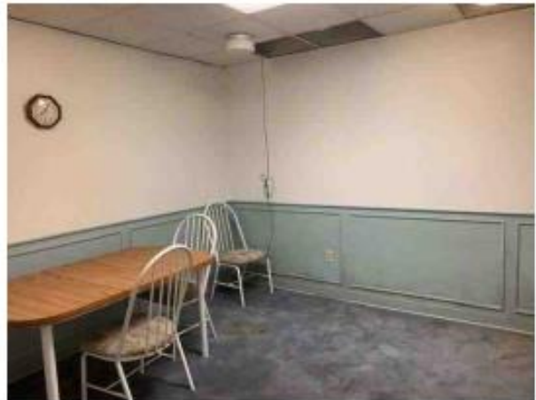
Break Room - Possible Mold/Ceiling Damage
