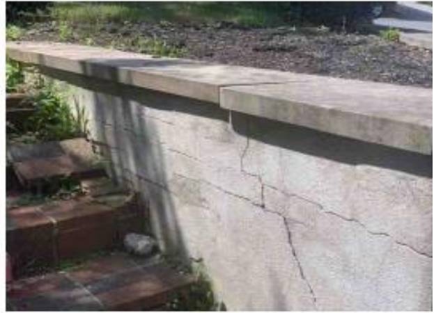
Deteriorated Steps and Retaining Wall
