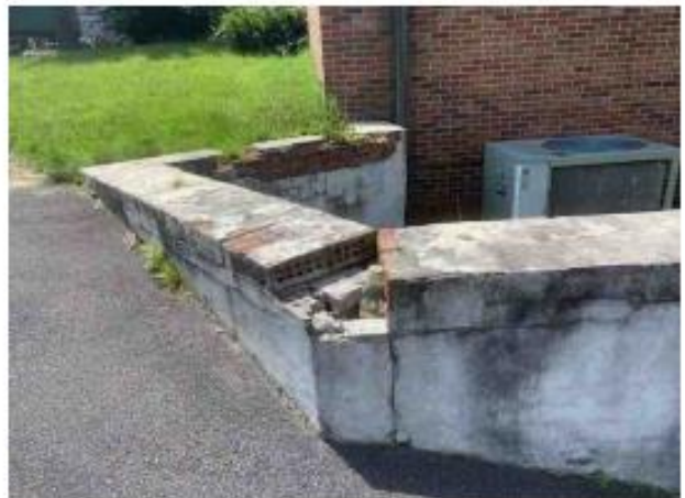
Damaged Retaining Wall
