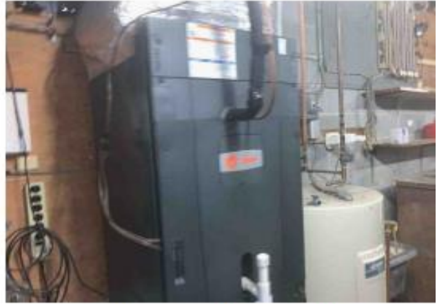
Furnace and Water Heater
