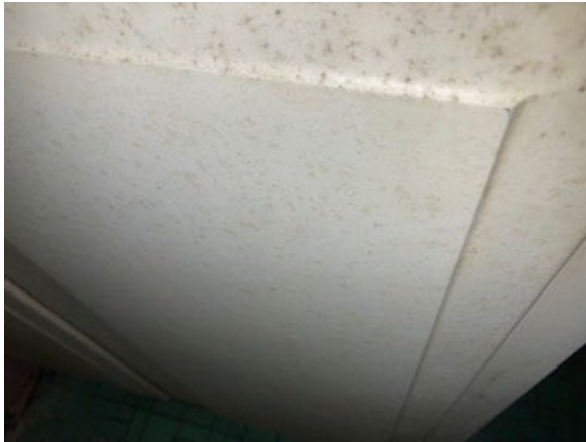
Probable mold on cabinet.
