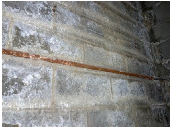
Efflorescence on furnace room wall.
