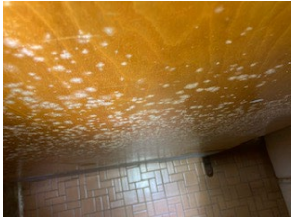
Probable mold on door.
