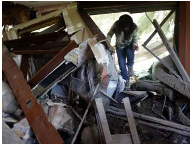
Figure 28. Landslide Damage to a Historic Jordan Brewery (Feyder, 2014)
