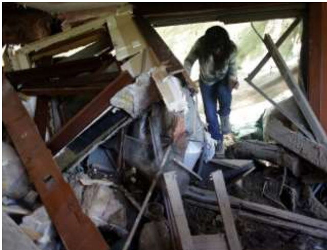
Figure 32. Landslide Damage to a Historic Jordan Brewery (Feyder, 2014)
