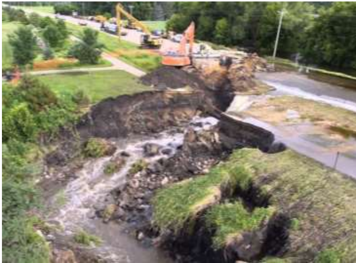
Figure 18. Flood Damage on County Road 16, Shakopee, June 27, 2014 (Noess, 2014)
