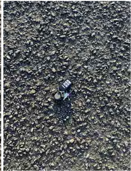
High Severity Raveling
