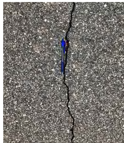
Low Severity Transverse Cracking
