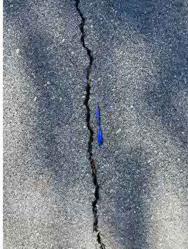
Medium Severity Transverse Cracking
