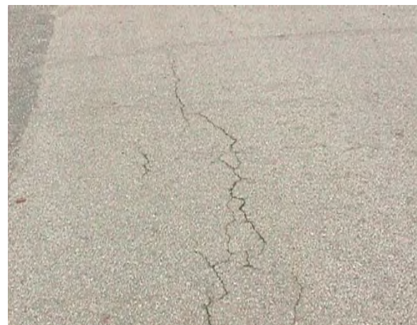
Low Severity Fatigue Cracking
