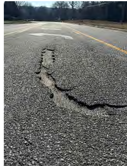
Medium Severity Pothole
