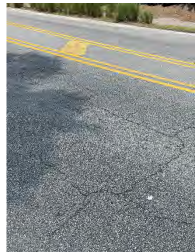
Low Severity Block Cracking
