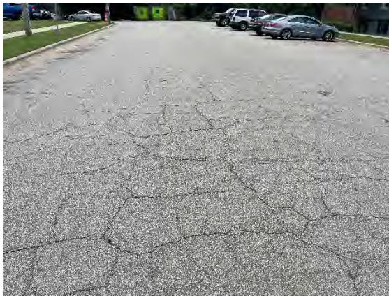
Medium Severity Block Cracking
