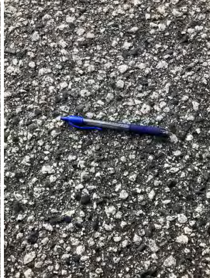
Medium Severity Raveling
