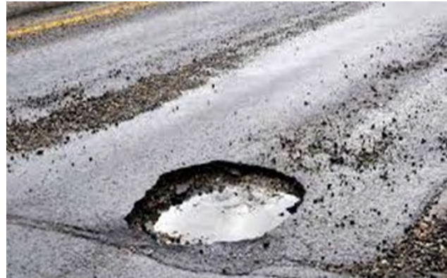
High Severity Pothole
