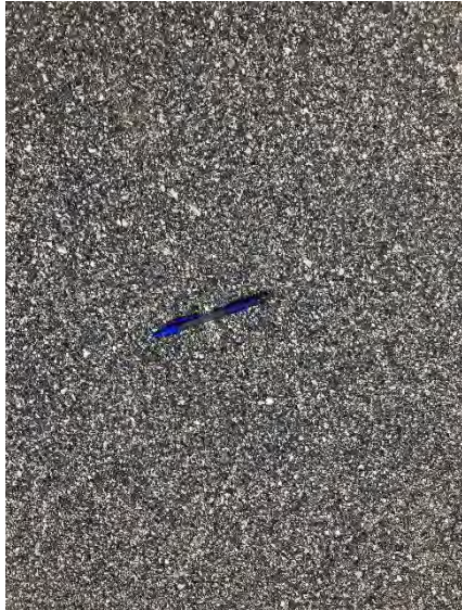
Low Severity Surface Defects
