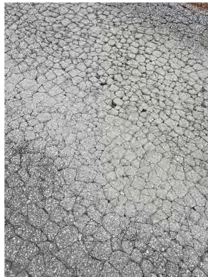
High Severity Fatigue Cracking
