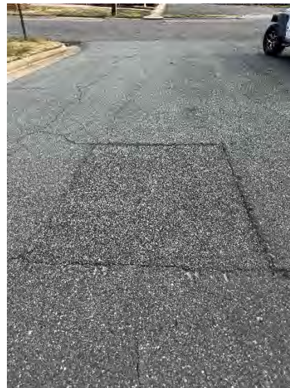
Low Severity Patch
