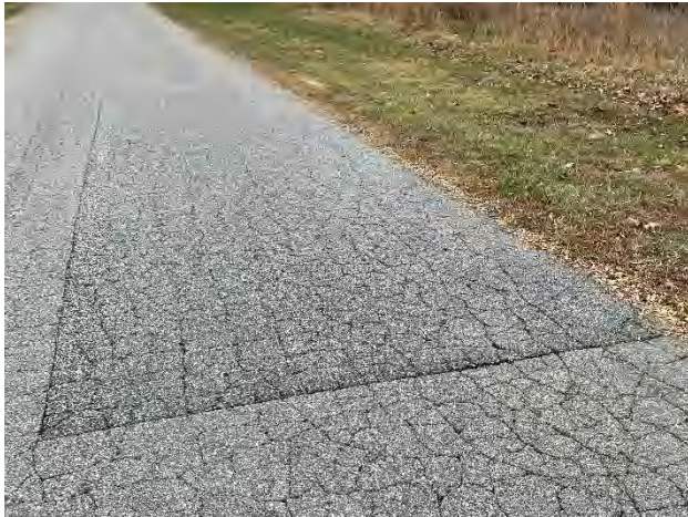
Medium Severity Patch
