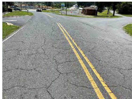
High Severity Block Cracking
