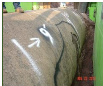
Damage concentrated in 9' section
