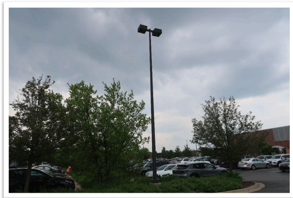
Photograph 34: Typical view of pole light
