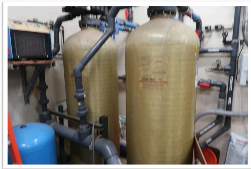
Photograph 20: Typical view of irrigation system sand filters
