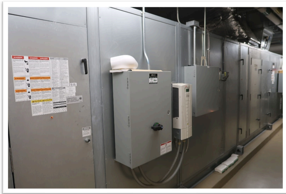
Photograph 19: Typical view of air handler
