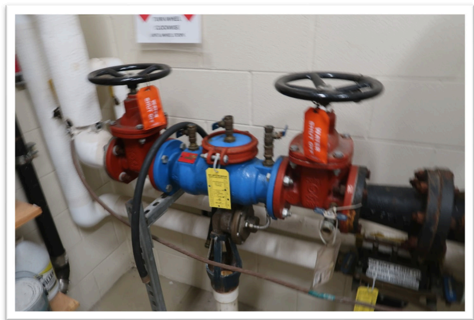
Photograph 22: Typical view of backflow preventer
