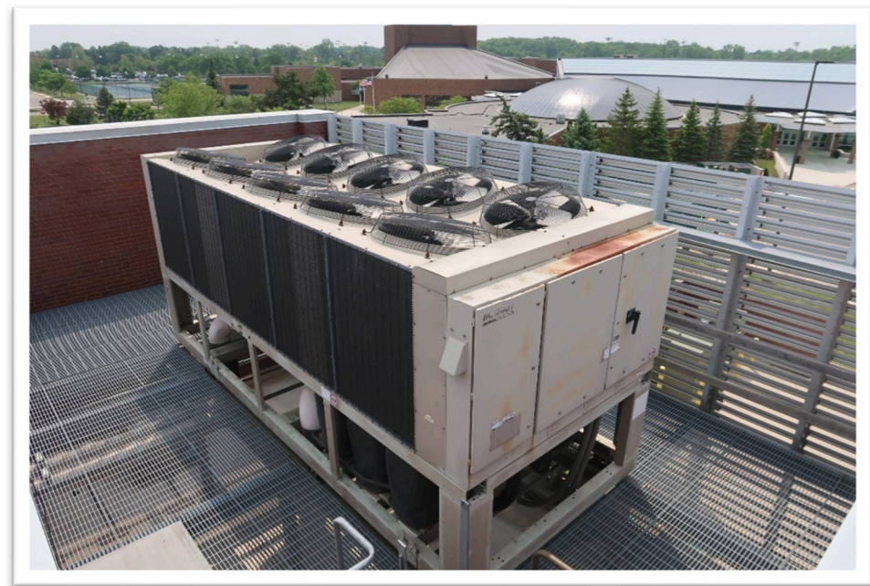
Photograph 18: Typical view of 60 ton chiller
