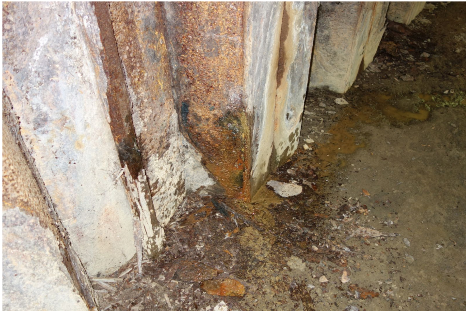
South Abutment Sheeting Section Loss and Rusting
