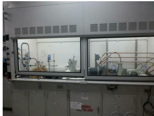
Typical LAB Hood with Sash Control
