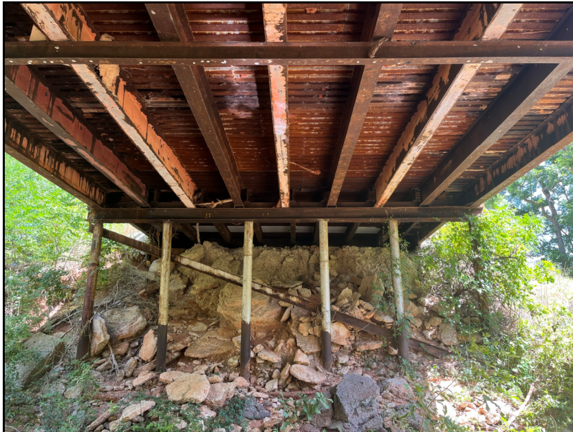
Figure 4 – Rust and Pitting in the Steel Girders and Stay-In-Place Forms
