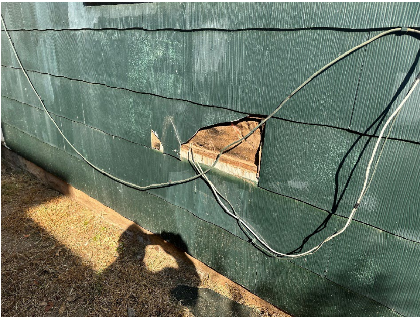
Damaged siding on south side of home
