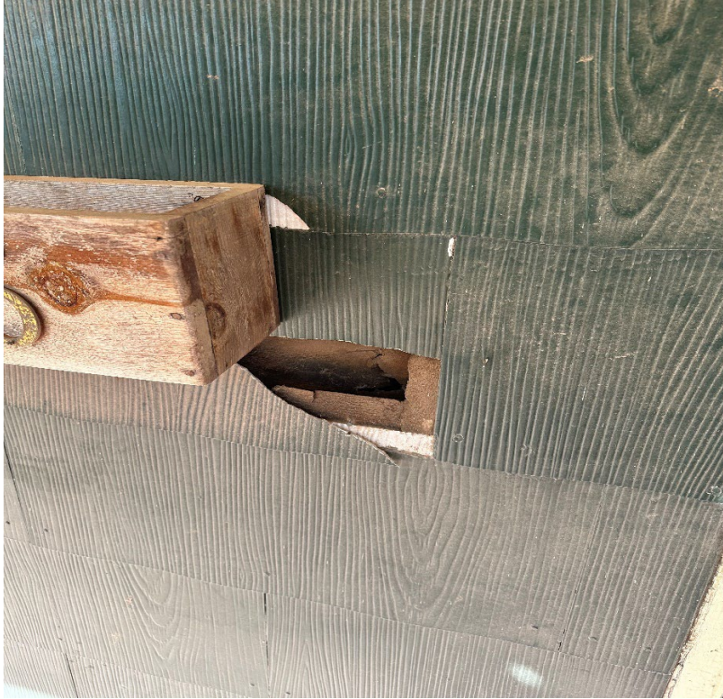
Damaged siding on porch
