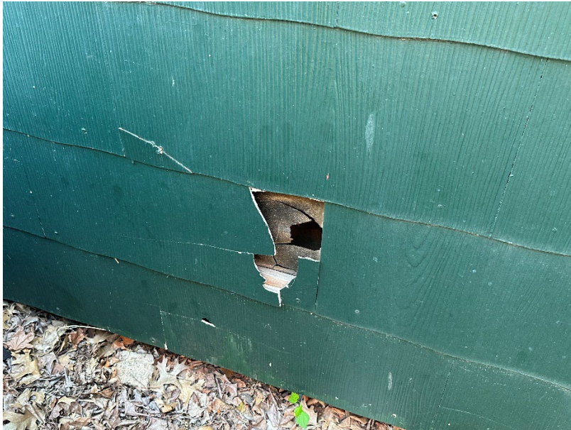
Damaged siding on north side of home
