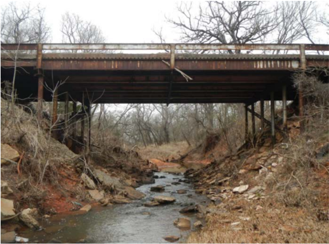
60 th Ave NE Bridge over Rock Creek (located north of Rock Creek Rd).
