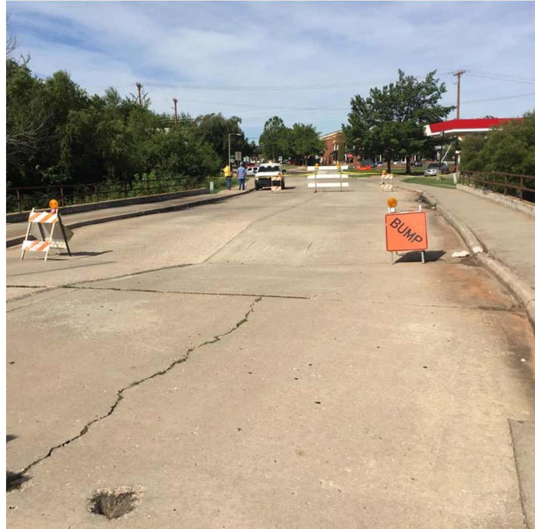
HavenBrook Bridge Failure – September 26, 2016
