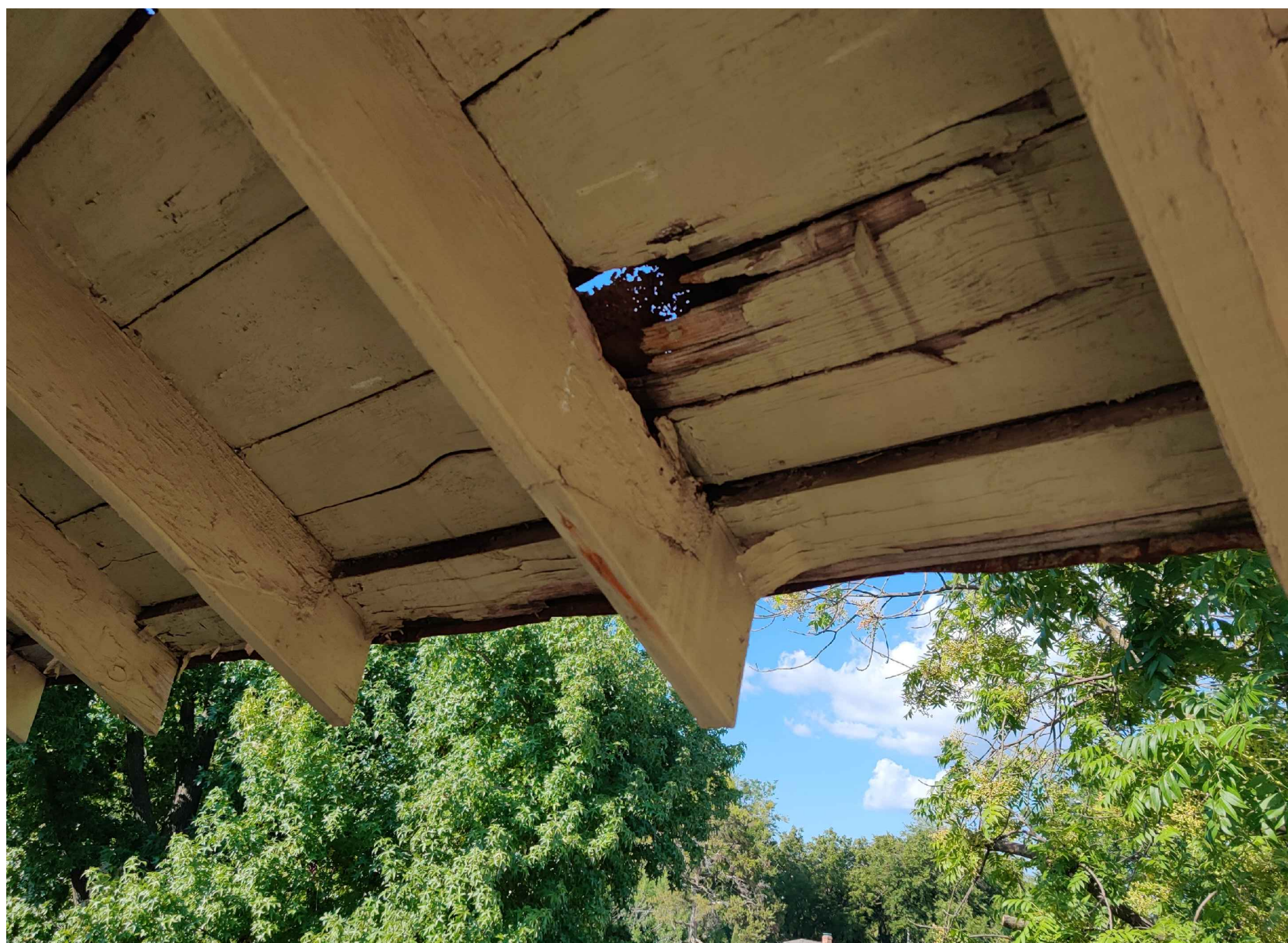
PHOTO- FAILURE OF ROOF AND DECK
