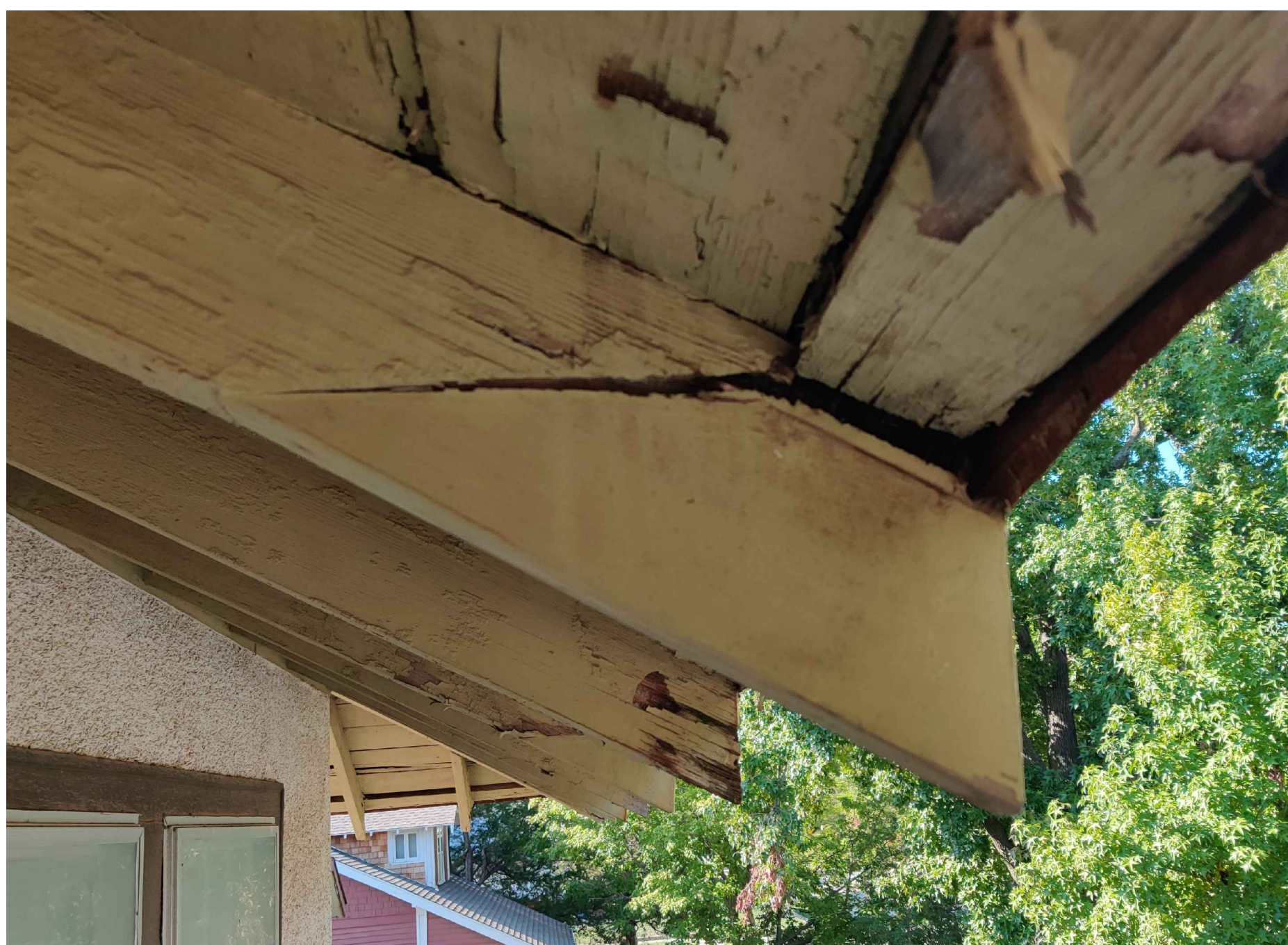
PHOTO- FAILURE OF SPLICED RAFTER TAIL
