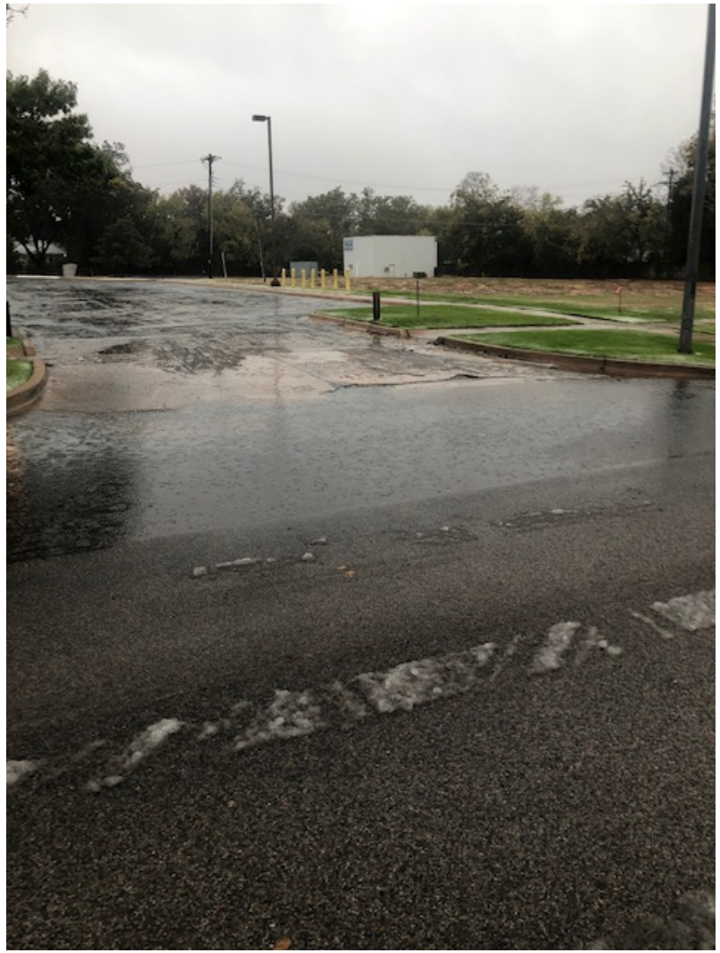
Water ponding in gutter line during rain events
