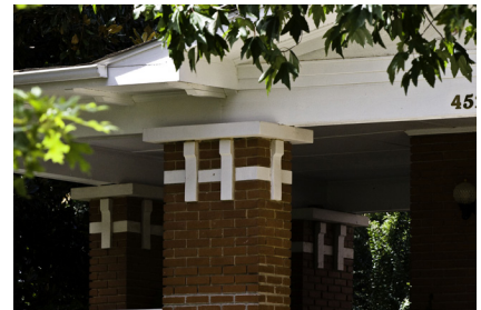
These brick columns on a Craftsman structure also include cast concrete capitals and details.
