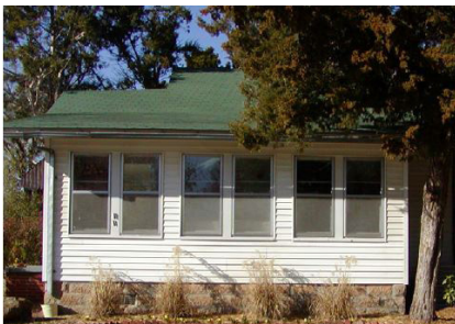
Original window placement often maximizes passive solar as in this south-facing elevation with three pairs of windows.
