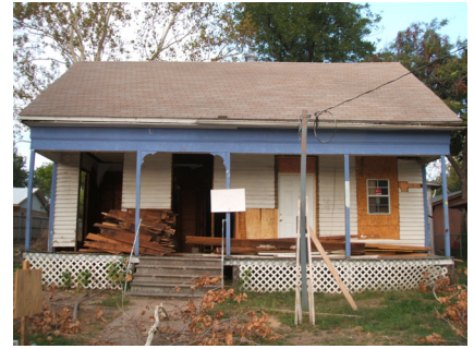
Maintain historic buildings by repairing limited areas of damage rather than the whole building.
