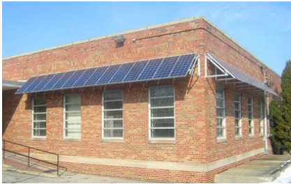
Solar panels, which also serve as awnings, were installed in secondary locations on the side and rear of this historic post office and cannot be seen from the front of the building. (Source: NPS)
