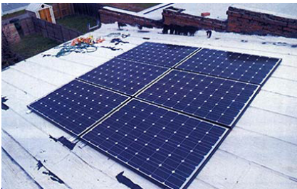
Solar panels were installed appropriately on the rear portion of the roof on this historic house that are not visible from the primary elevation. (Source: NPS)
