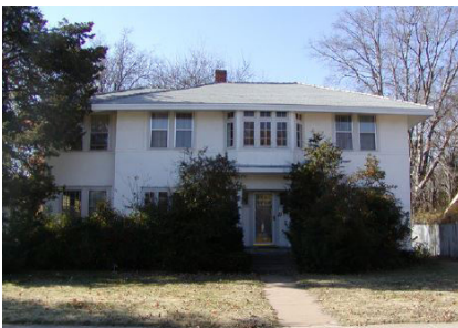
A mixture of hung and casement windows characterize this unusual Italian Renaissance structure in the Chautauqua District.
