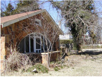
This bungalow has a full-width porch with stone cladding and an unusual elliptical opening.
