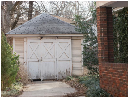
A pyramidal roof was common on single car garages built in the 1920s.
