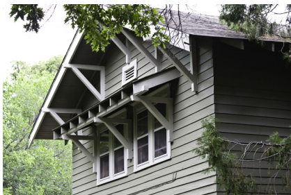
A shed roof supported by brackets provides shade, decorative detail, and support on a Craftsman structure.
