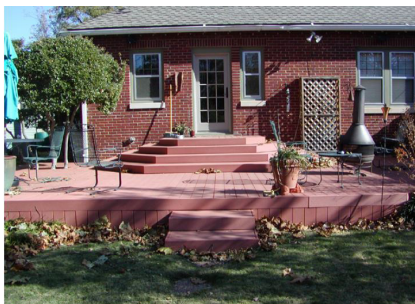
Alternative building materials are possible when decks are installed in an inconspicuous location such as the rear yard of an interior lot.
