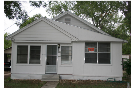
Wood windows should be repaired and not replaced with aluminum frame windows.
