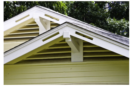
Attic ventilation is accomplished through the use of decorative wooden louvers in a roof gable.
