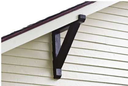
Wood brackets, sometimes known as knee braces, are common decorative support elements on bungalows.
