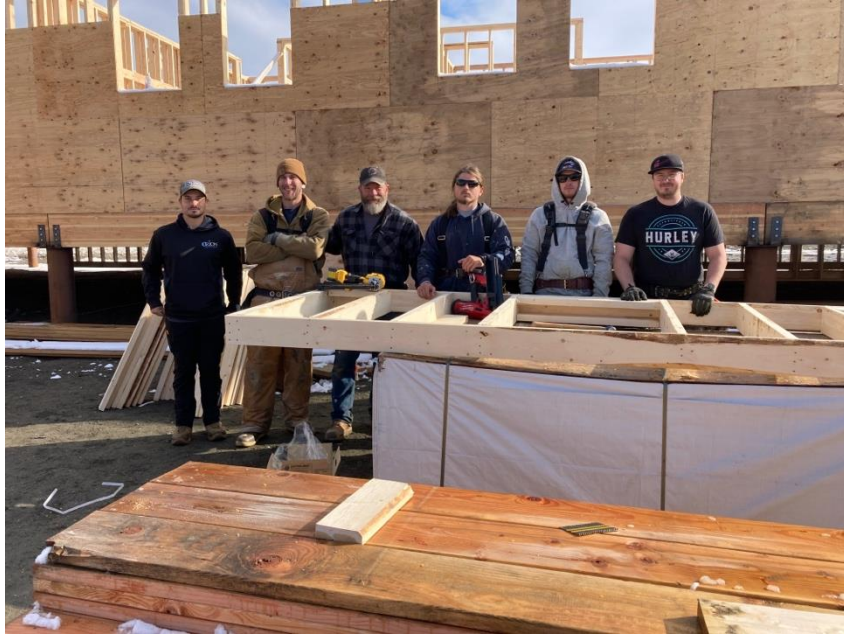
Pictured here is the first crew that framed the structure. Devon is the fourth from the left. (Not pictured is Mark Borghi, Project Superintendent)
