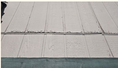
failed paint & water damage
