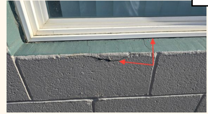
masonry sealant needed
