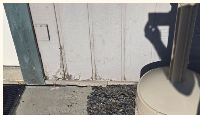
failed paint & water damage
