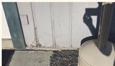
failed paint & water damage
