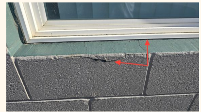
masonry sealant needed
