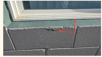
masonry sealant needed
