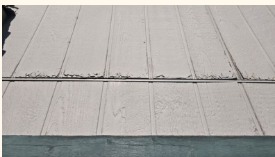
failed paint & water damage
