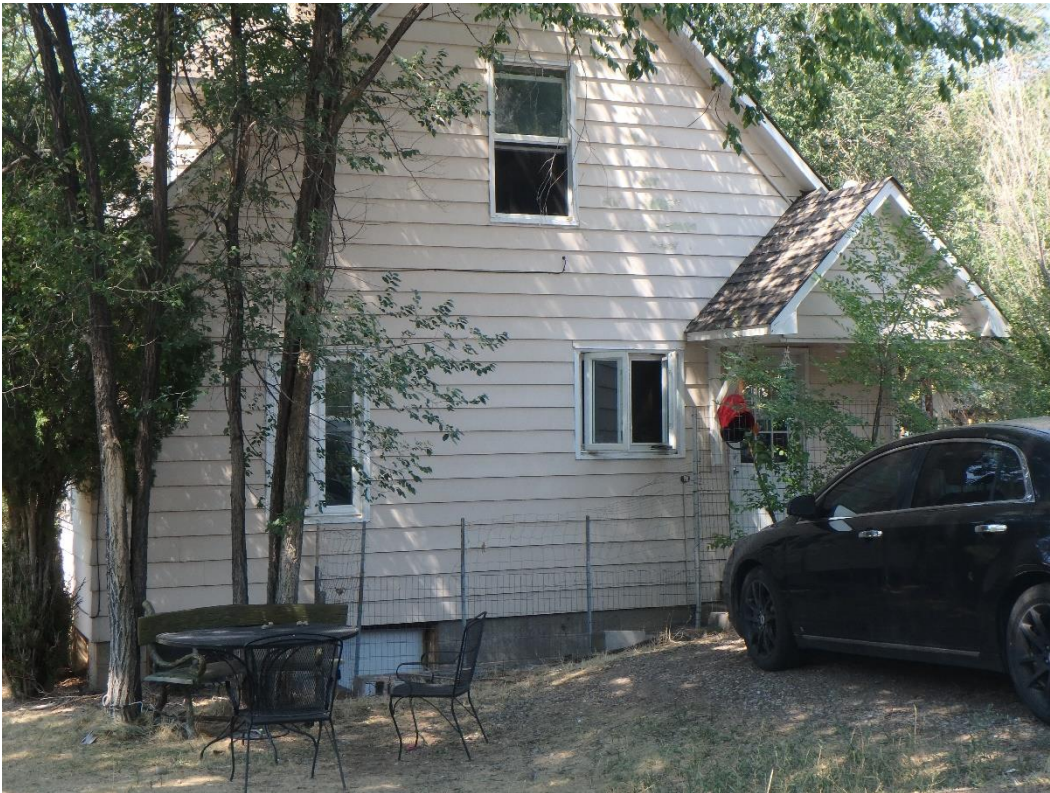
Photo Number: 5GF.5924_4 Description: Looking at the east elevation of the building. Date: 9/6/2022 View: Northwest
