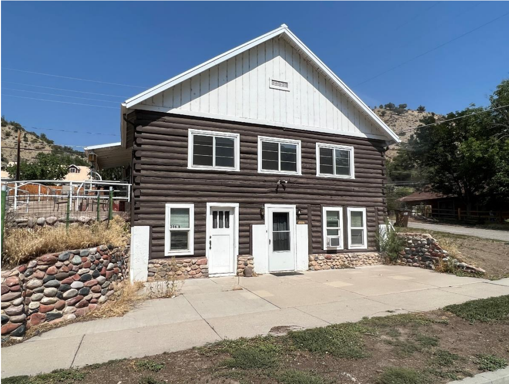
Photo Number: 5GF.5932_1 Description: Looking at the south elevation of the building. Date: 9/6/2022 View: Northeast
