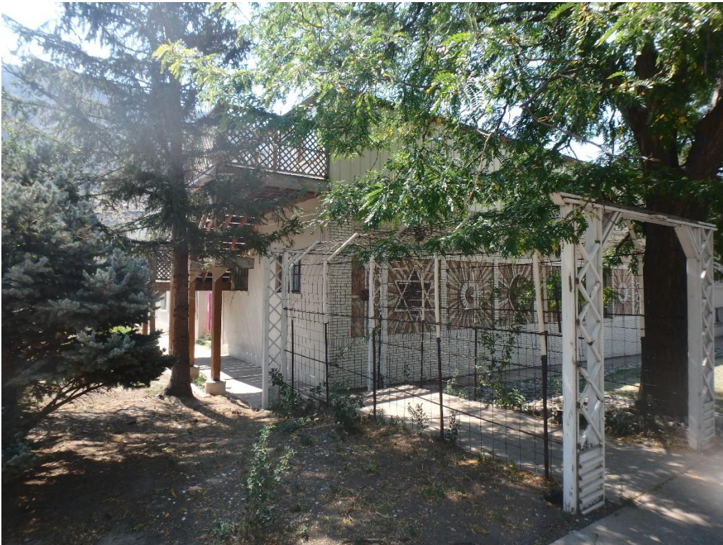
Photo Number: 5GF.2369_4 Description: Looking at the corner of the east elevation and the primary (north) elevation. Note the staircase leading to the second level addition to the building. Date: 9/6/2022 View: Southwest
