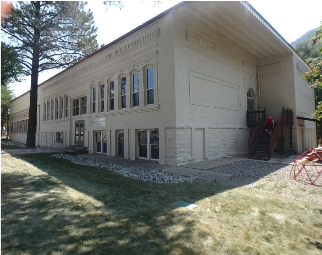
Photo Number: 5GF.2369_1 Description: Looking at the primary (north) and west elevations of the building. Note the several ornate brickwork features along the facade. Date: 9/6/2022 View: Southeast
