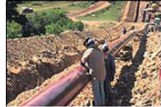
Figure 26: Natural Gas pipeline.
