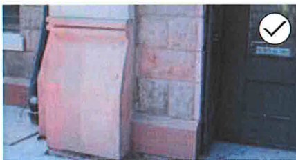
33. If necessary, repair a foundation wall using new material that is similar in character to the original. The foundation illustrated in the top image was patched with a consolidant that was tinted to match the existing pink sandstone, as illustrated below.
