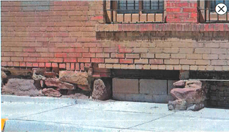
31. Do not allow an original foundation to fall into disrepair.
