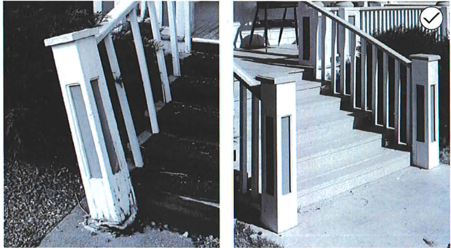
44. Maintain and repair historic porch and stoop components, finishes and details. For example, this deteriorated porch railing illustrated at left has been restored to its original condition, as illustrated at right.
