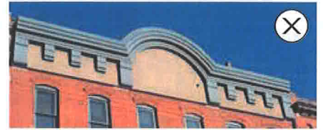
27. Avoid removing or covering original roof materials and features that are in good condition. The original brick parapet on the building illustrated above is covered with a stucco and wood replacement that does not match the original.
