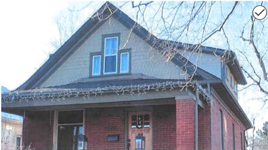
30. Design a dormer to be subordinate to the overall roof mass and in scale with those on similar historic structures. The dormer is set back behind the overhanging roof eave and the adjacent brick wall plane.
