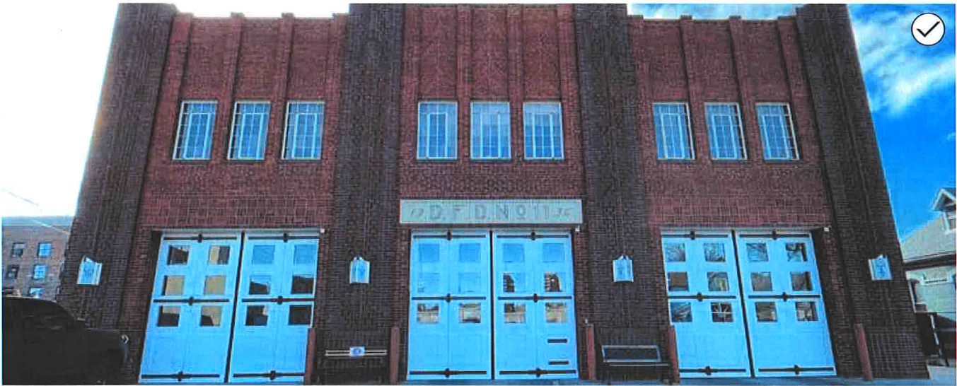
25. Replacement doors to match the design of the original historic doors. Original historic hardware reused.
