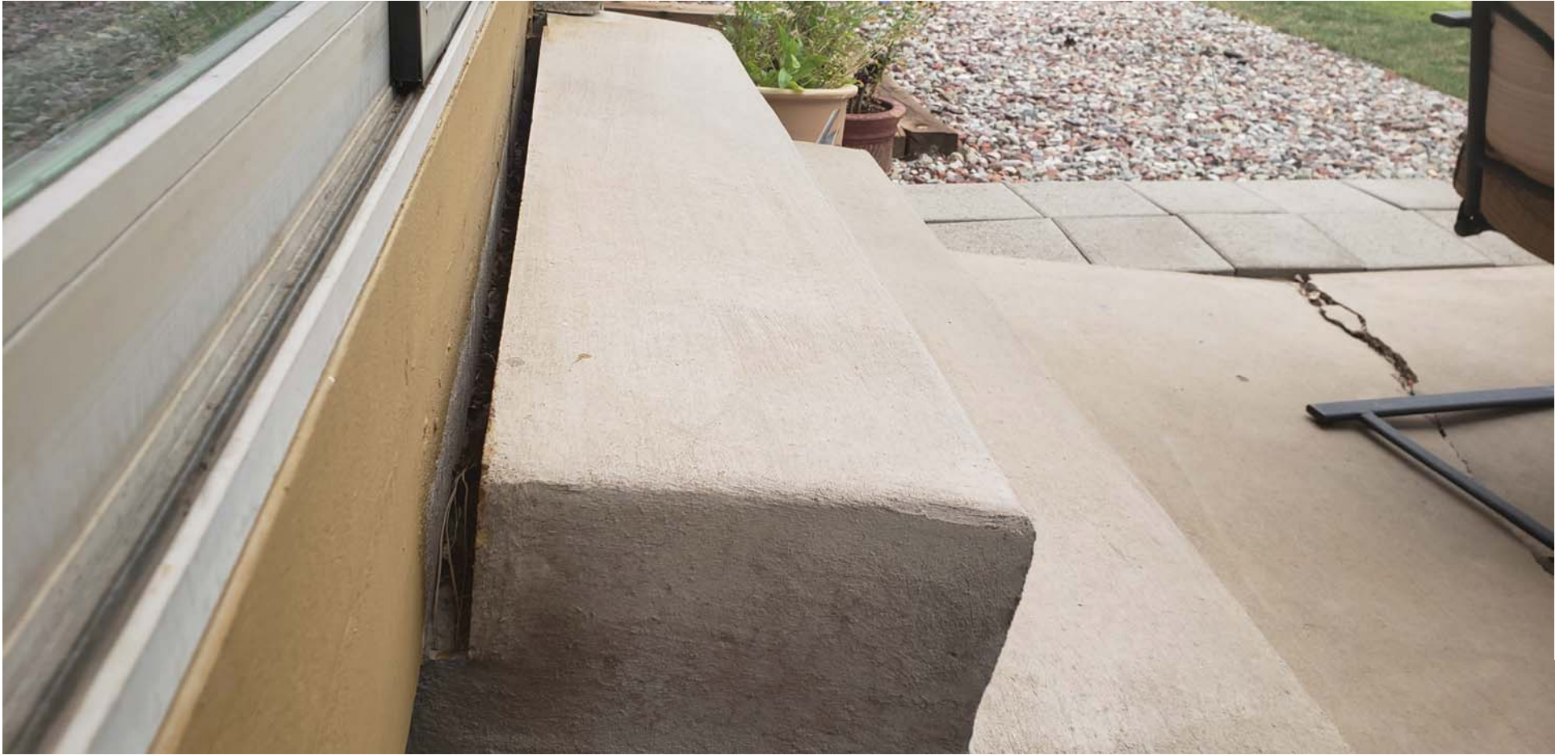
Stairs Pulling Away
