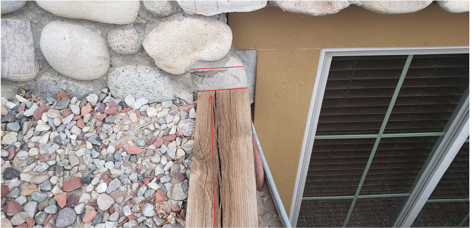
Window Well Settlement
