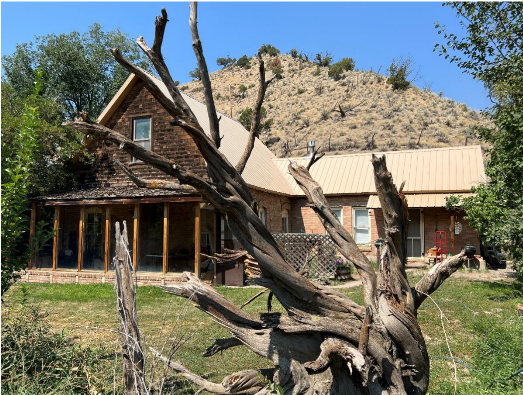
Photo Number: 5GF.5943_2 Description: Looking at the entire facade of the primary (south) elevation. Note the wood shingle exterior in the gable end while brick masonry cladding encompasses the right side of the building. Date: 9/6/2022 View: Northwest
