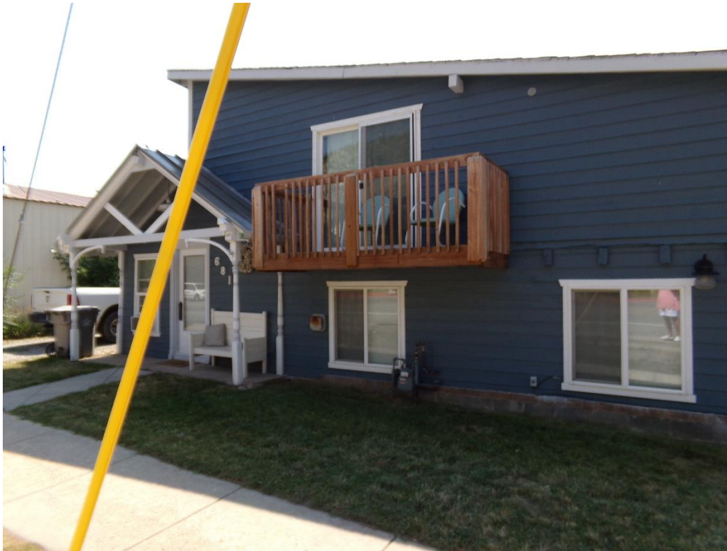
Photo Number: 5GF.5899_1 Description: Looking at the primary (north) elevation of the building. Date: 9/6/2022 View: Southeast
