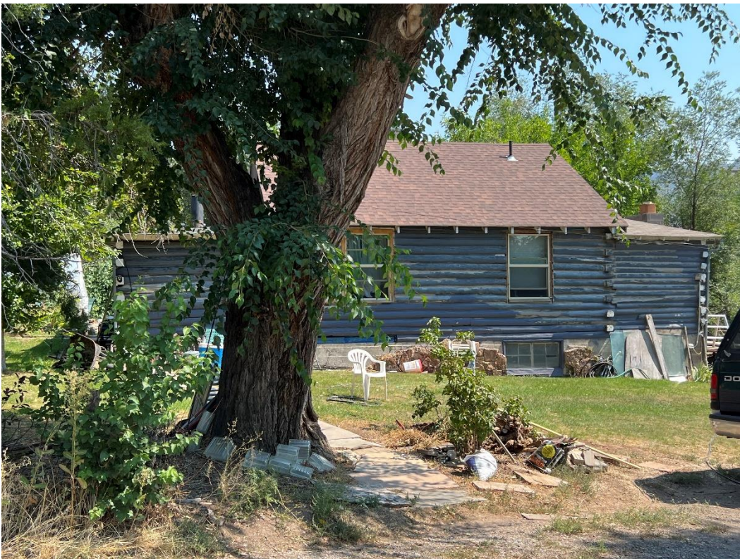
Photo Number: 5GF.5939_4 Description: Looking at the west elevation of the building. Note the CMU block chimney along the south elevation of the building. Date: 9/6/2022 View: East
