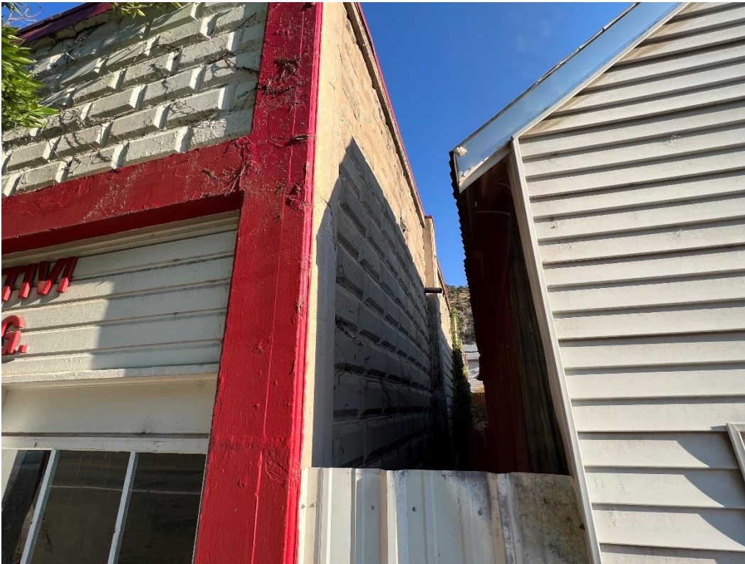
Photo Number: 5GF.2373_5 Description: Looking at the east elevation of the building. Date: 9/6/2022 View: North
