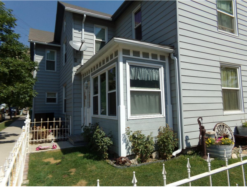
Photo Number: 5GF.5900_3 Description: Looking at the west and south elevations of the building. Date: 9/6/2022 View: Northeast
