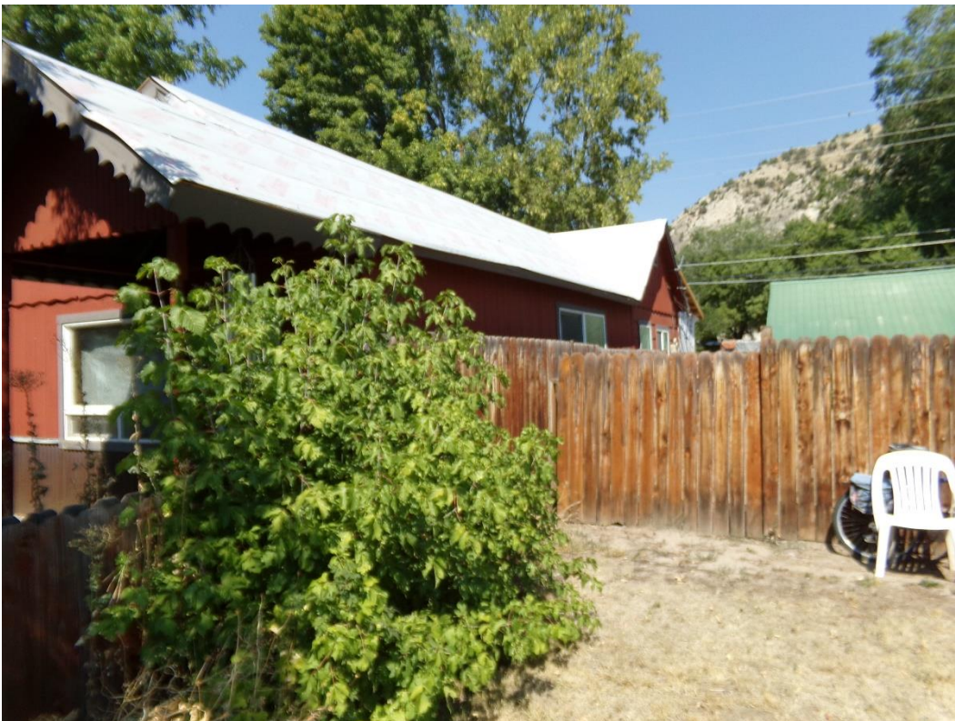
Photo Number: 5GF.5895_2 Description: Looking at the east elevation of the building. Date: 9/6/2022 View: Northwest
