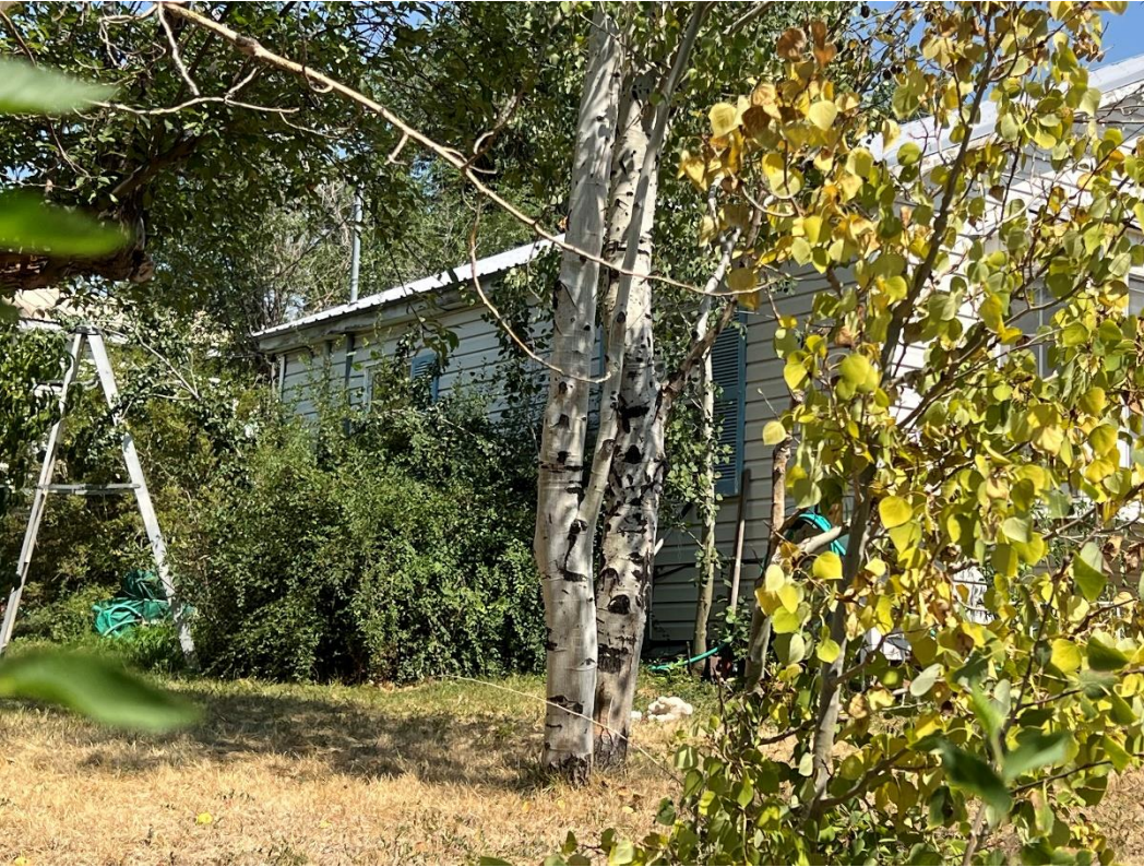
Photo Number: 5GF.5929_3 Description: Looking at the west elevation of the primary building. A majority of the elevation is obscured by vegetation. Date: 9/6/2022 View: Northeast
