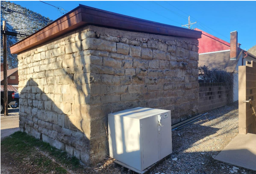
Photo Number: 5GF.2367_3 Description: Looking at the east and north elevations of the building. Date: 4/7/2023 View: Southwest
