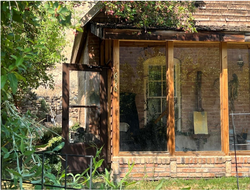
Photo Number: 5GF.5943_3 Description: A small glimpse of the west elevation of the building. Date: 9/6/2022 View: Northeast
