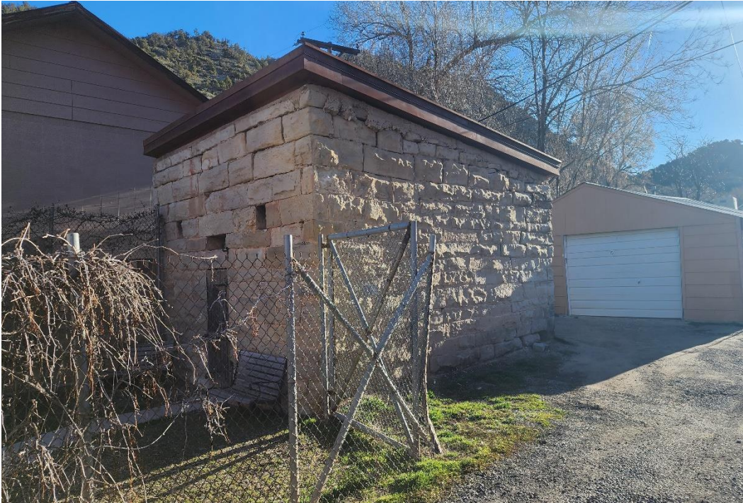
Photo Number: 5GF.2367_1 Description: Looking at the primary (west) and south elevations of the building. Note the three vent openings above the main entryway. Date: 4/7/2023 View: Northeast
