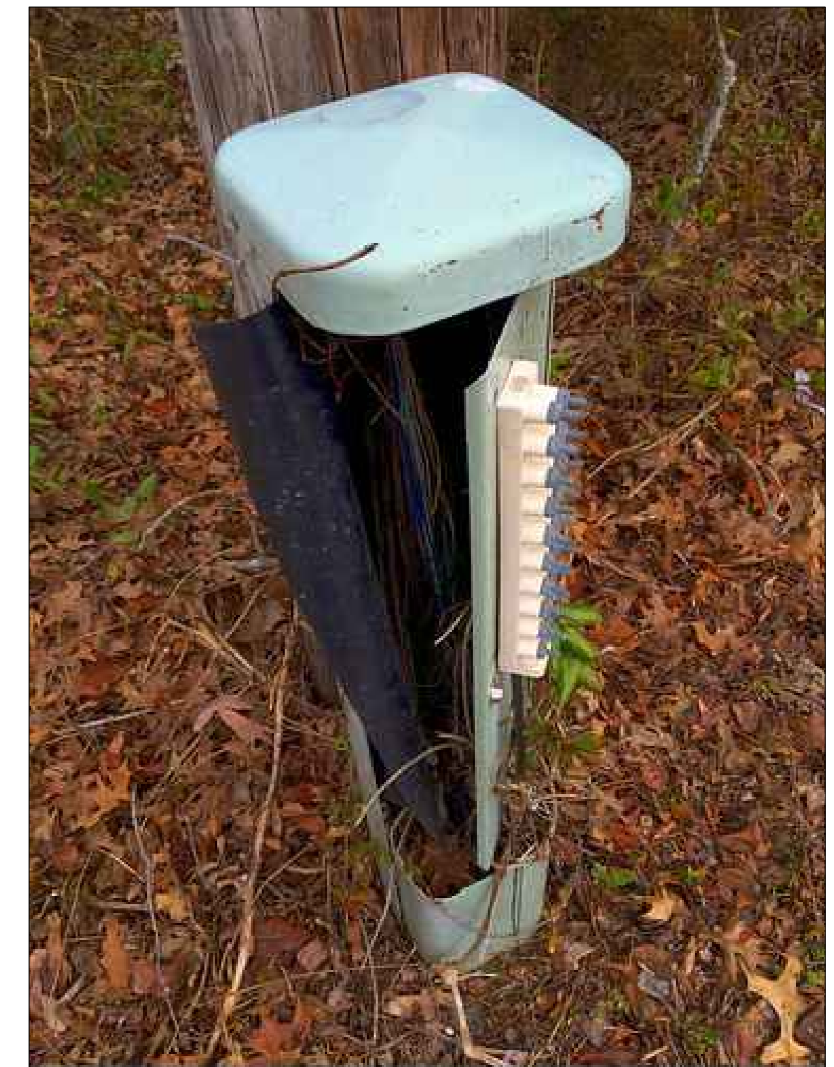
TELEPHONE PEDESTAL CONNECTION PHOTO
