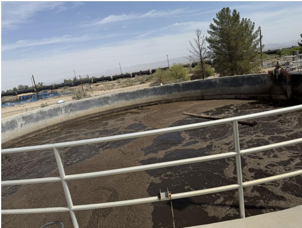
Figure 6. SBR No. 1 in operation at the time of inspection. Each SBR is designed to treat 600,000 gpd and provides equalization, aeration, and clarification into a single timed sequence in one reactor basin.
