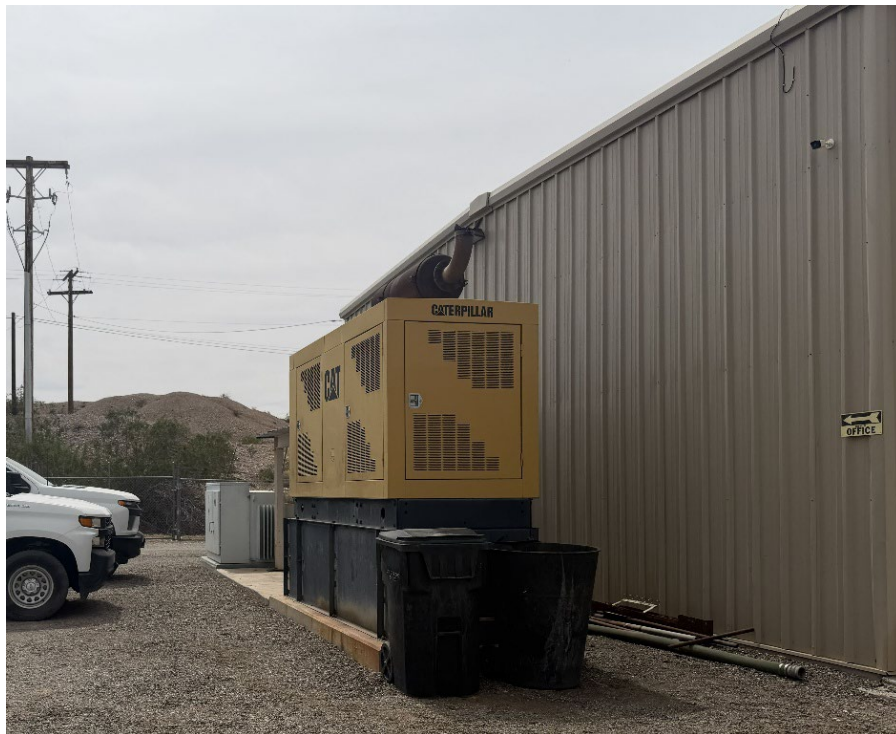
Figure 10. The emergency generator provides power to run the Facility in the event of a power outage.
