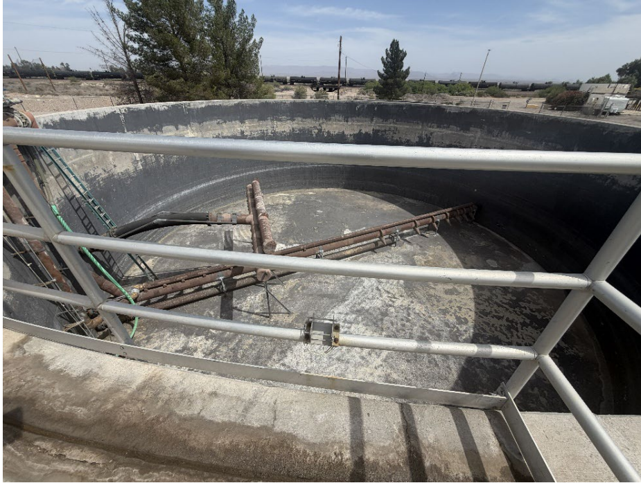
Figure 7. SBR No. 2 not in operation due to yearly maintenance. Typically, one SBR is in operation at a time.
