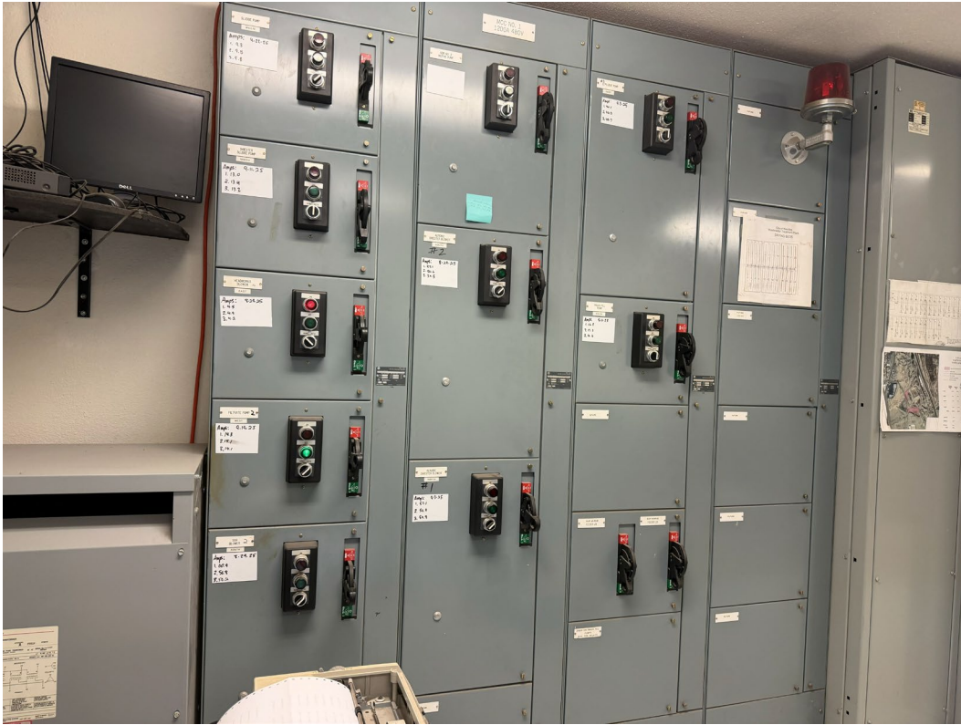
Figure 16 A motor control center located in the main office.
