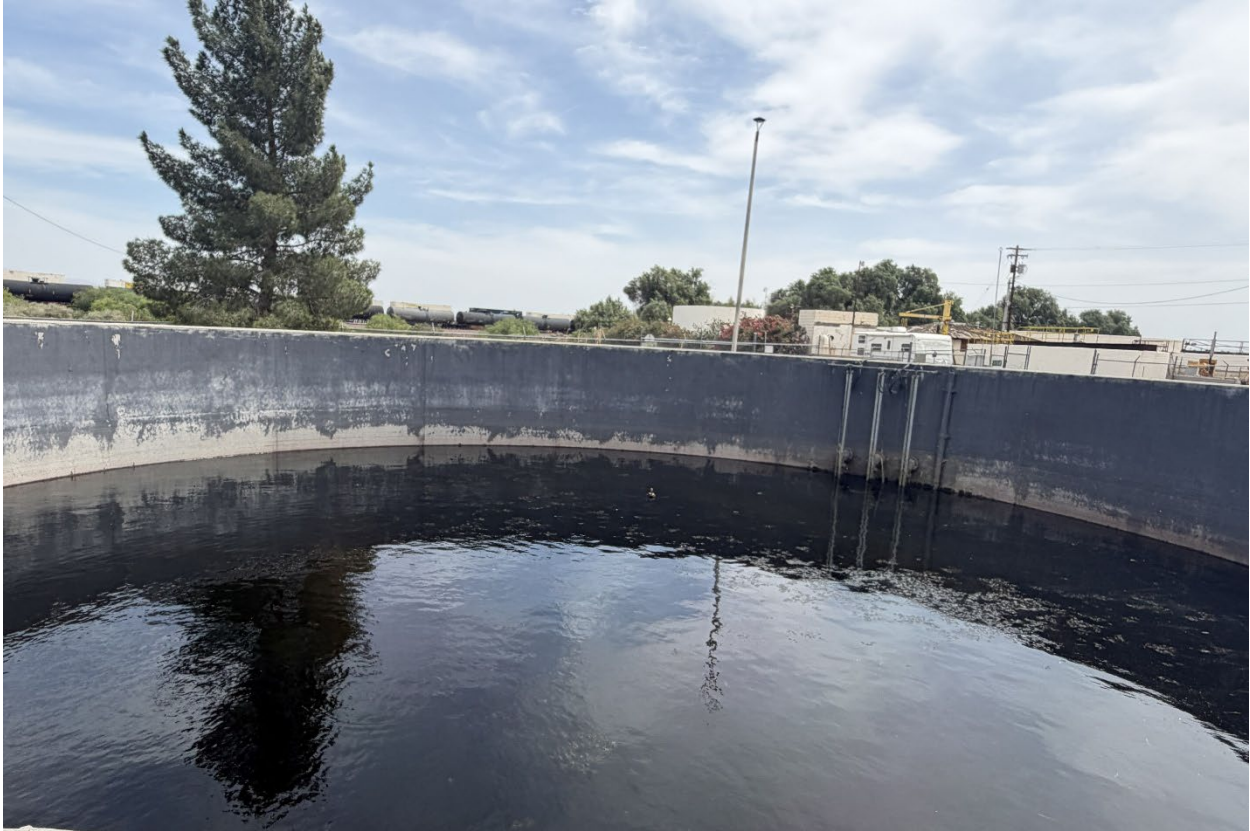
Figure 9. The effluent equalization basin stores treated wastewater. Treated wastewater from the effluent equalization basin is pumped to the evaporation/percolation ponds.
