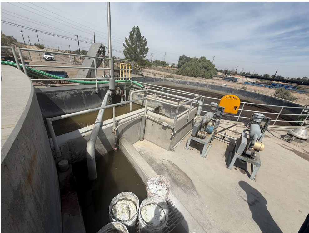
Figure 4 The aerated grit chamber that utilizes an airlift pump that operates 24 hours a day. Grit is collected in 5-gallon buckets, and lime is placed on top to help limit vectors and odors.
