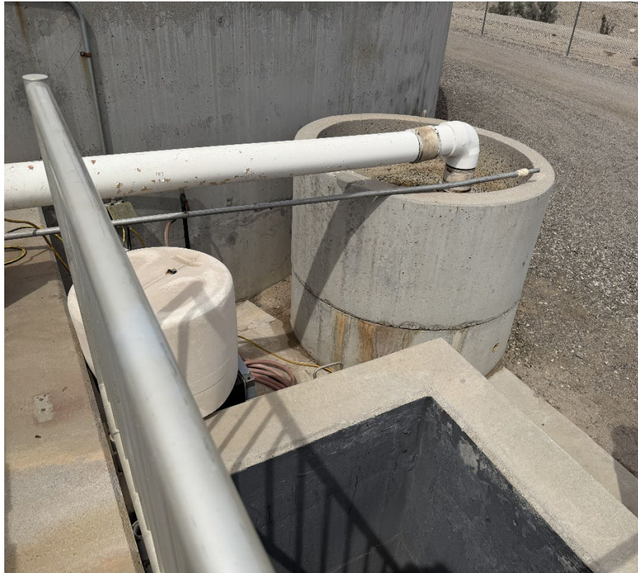
Figure 8. The effluent wet well shown in the foreground. Effluent samples are taken from the effluent wet well using an automated composite sampler located to the left. In the background a wood chip basin is used for odor control.
