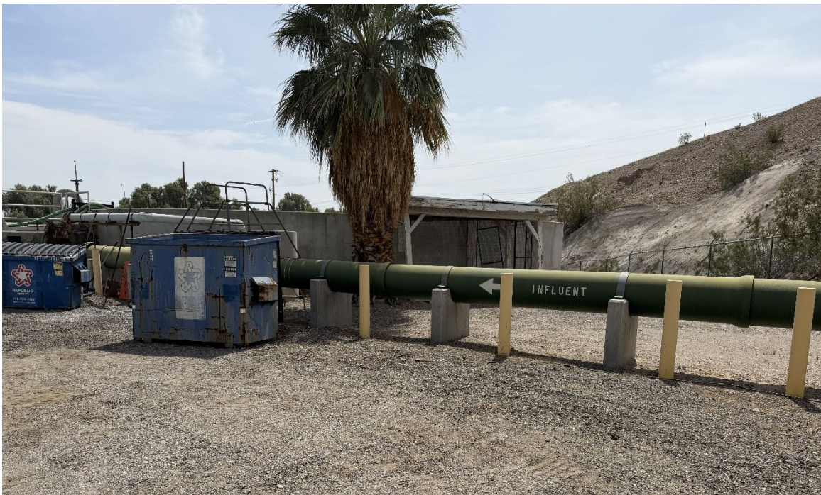
Figure 2. The influent wastewater pipeline routes wastewater from the sewer collection system to the treatment plant and is clearly labeled. The influent pipeline is located on the east side of the Facility.
