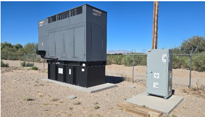
Phase 4A: Emergency Generator at Well 11
