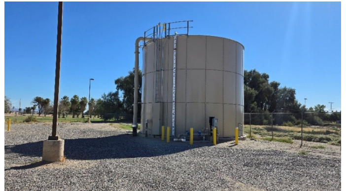
Backwash Water Tank
