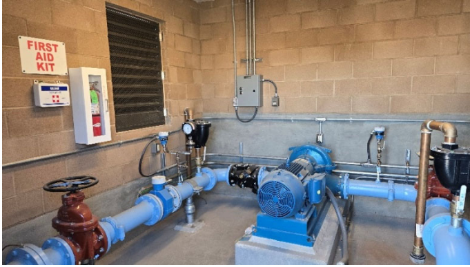
Booster Pumps and Plumbing
