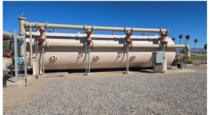
Pressure Filtration System
