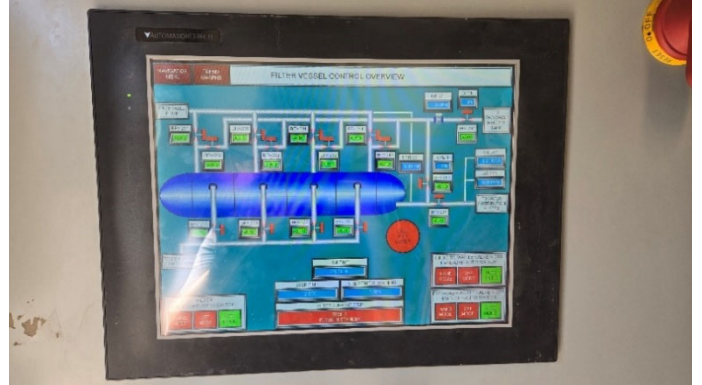
Control Panel Display for Filtration System
