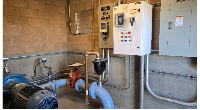
Control and Power Panels
