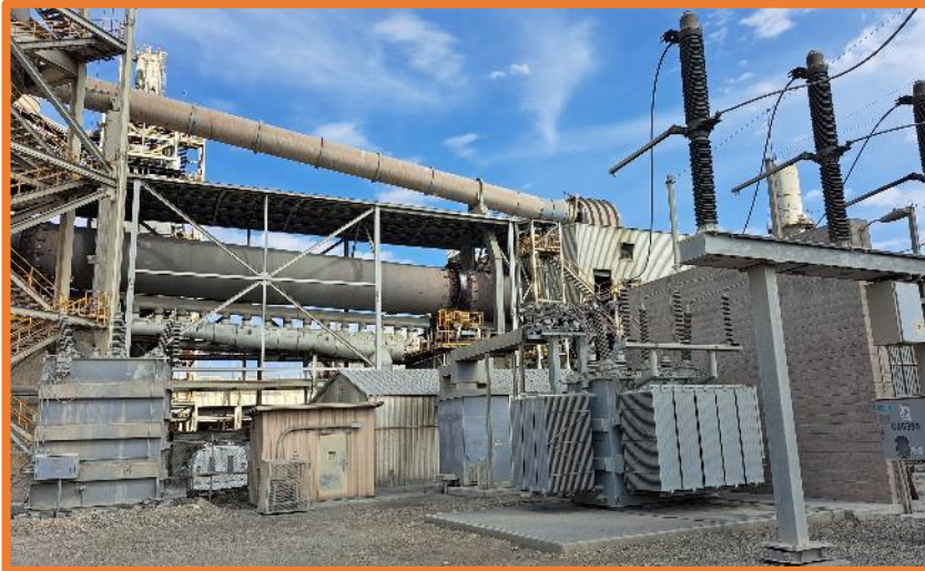
Industrial Substation PWT Replacement, TXI T1 ($1.1M)
